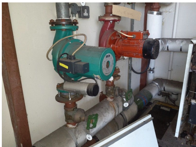
Sample No: 23/4/B/25/JPS19 2.03 Boiler Room Pipework Flanges Gaskets containing: Chrysotile
