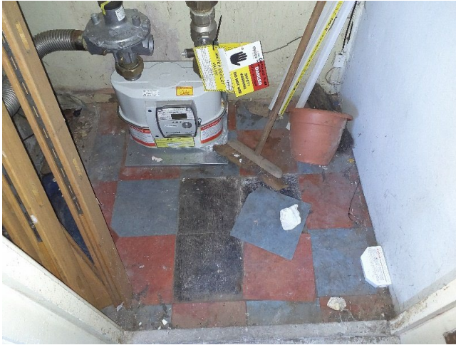
Sample No: Refer to Sample 23/4/B/25/JPS6 G.05 Store Room Floor Area Vinyl Floor Tiles and Bitumen Adhesive containing: Chrysotile (In both tile and bitumen)
