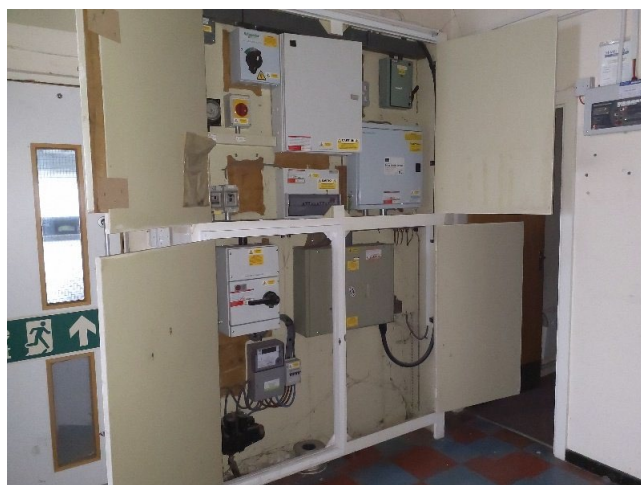
G.02 Warehouse - Electrics Live at Time of Survey
