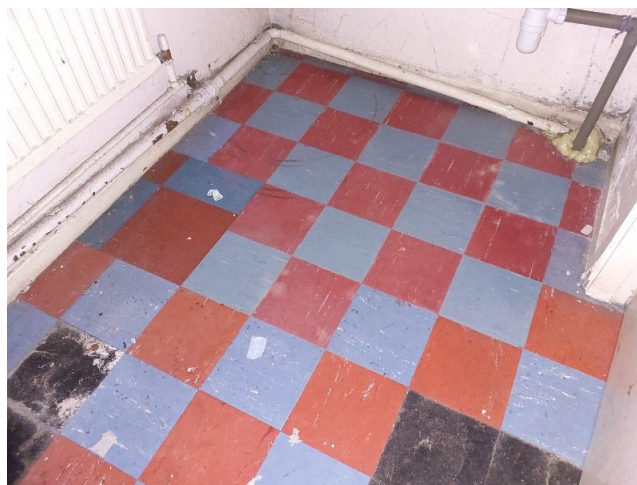
Sample No: Refer to Sample 23/4/B/25/JPS6 G.07 Gents Toilet Floor Area Vinyl Floor Tiles and Bitumen Adhesive containing: Chrysotile (In both tile and bitumen)
