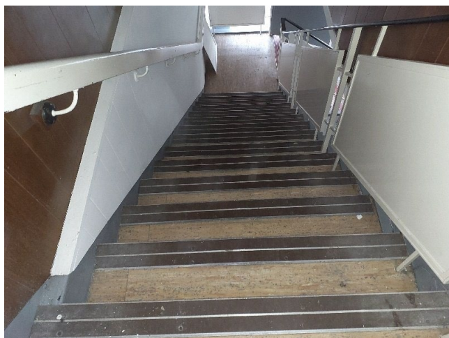
Sample No: Refer to Sample 23/4/B/25/JPS4 1.01 Stairs / Landing Stair Treads Vinyl Nosing containing: Chrysotile
