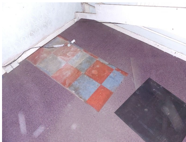
Sample No: Refer to Sample 23/4/B/25/JPS6 G.04 Office Floor Area Vinyl Floor Tiles and Bitumen Adhesive containing: Chrysotile (In both tile and bitumen)
