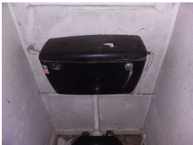
Sample No: 23/4/B/25/JPS10 G.06 Ladles Toilet Cistern Thermoplastic containing: Amosite
