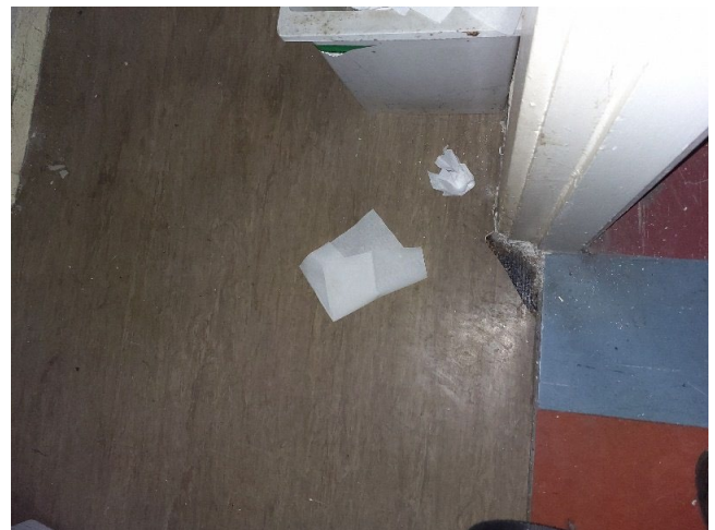
Sample No: 23/4/B/25/JPS9 G.06 Ladles Toilet Floor Area Vinyl Floor Covering & Bitumen Adhesive containing: Chrysotile (In bitumen only)
