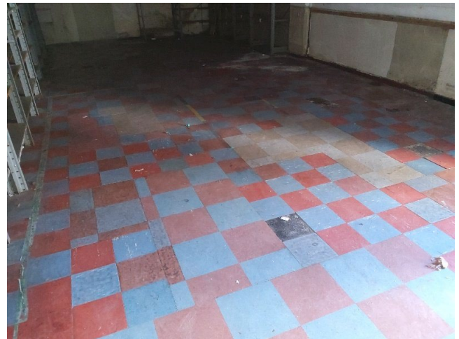
Sample No: 23/4/B/25/JPS6 G.03 Warehouse Floor Area Vinyl Floor Tiles and Bitumen Adhesive containing: Chrysotile (In both tile and bitumen)
