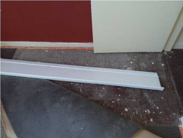
Sample No: Refer to Sample 23/4/B/18/JPS6 1.03 Lounge Below Carpet Vinyl Floor Tiles and Bitumen Adhesive containing: Chrysotile (In both tile and bitumen)
