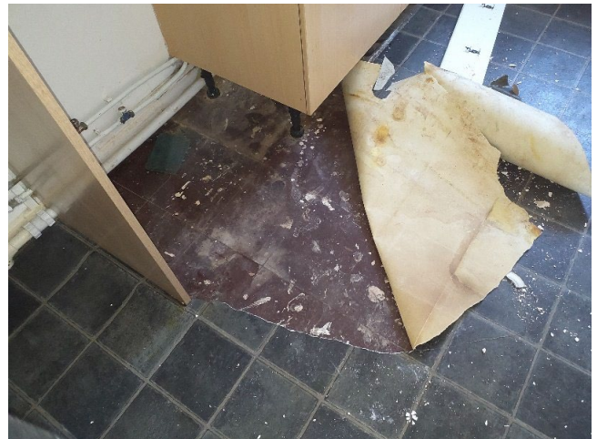
Sample No: Refer to Sample 23/4/B/18/JPS6 1.05 Kitchen Below Modern Vinyl Flooring Vinyl Floor Tiles and Bitumen Adhesive containing: Chrysotile (In both tile and bitumen)
