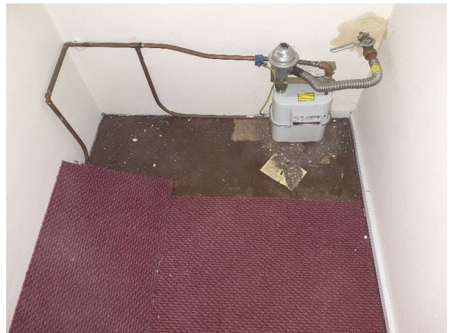
Sample No: Refer to Sample 23/4/B/18/JPS6 1.02 Store Room Below Carpet Vinyl Floor Tiles and Bitumen Adhesive containing: Chrysotile (In both tile and bitumen)
