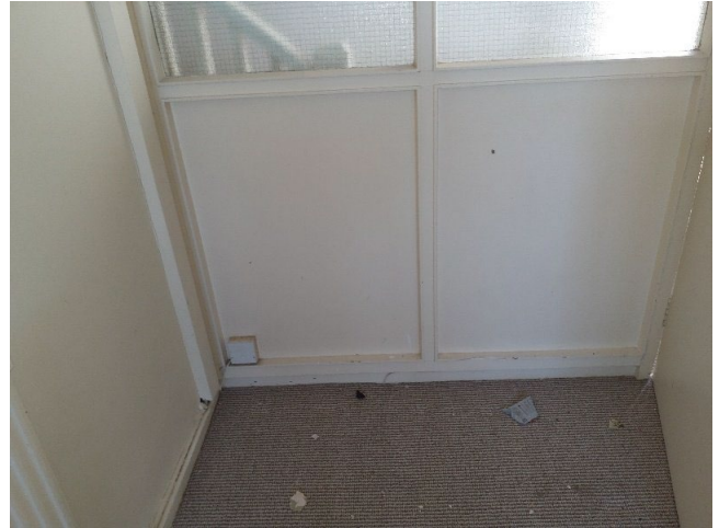
Sample No: Refer to Sample 23/4/B/18/JPS7 1.03 Lounge Combination Frame Spandrel Panels Composite Board No Asbestos Detected
