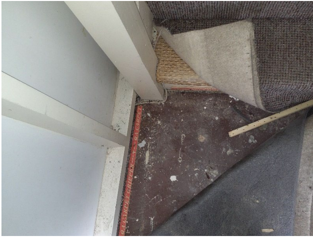
Sample No: 23/4/B/18/JPS6 1.01 Entrance Lobby Below Carpet Vinyl Floor Tiles and Bitumen Adhesive containing: Chrysotile (In both tile and bitumen)
