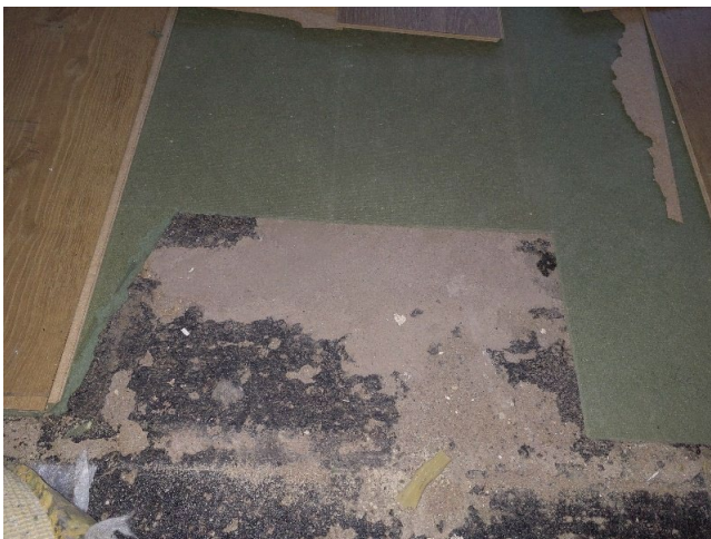
Sample No: 22/12/B/13/MAC2 1.01 Living room Floor below laminate flooring Residual bitumen adhesive containing: Chrysotile
