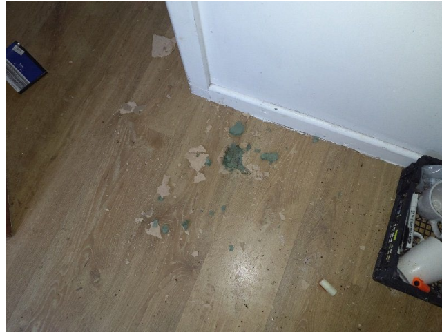
Sample No: Refer to Sample 22/12/B/13/MAC2 1.03 First floor entrance Floor below laminate flooring Residual bitumen adhesive containing: Chrysotile
