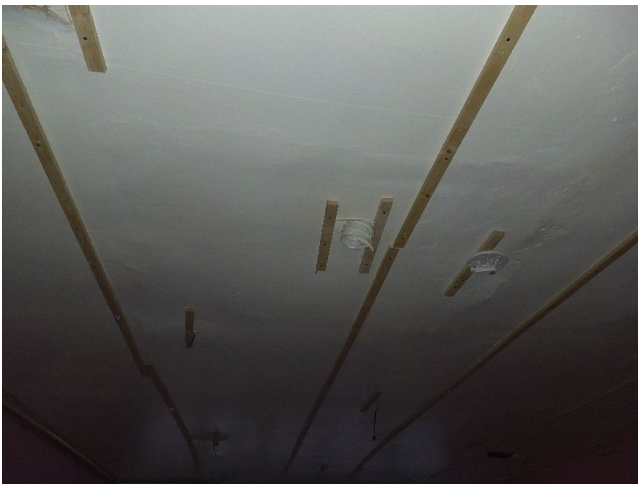
Sample No: 22/12/B/13/MAC1 G.01 Shop front Ceiling Fibreboard No Asbestos Detected
