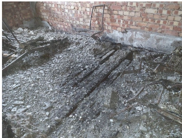
Fire damaged office 2.04
