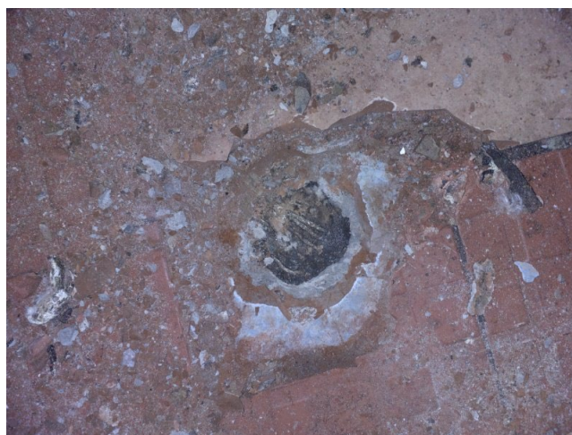
Sample No: 22/12/B/13/SAW1 G.01 Shop area Floor beneath screed Bitumen residuals containing: Chrysotile
