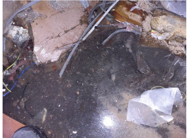
Sample No: Refer to Sample 22/12/B/13/SAW1 G.03 Under stairs cupboard Floor beneath screed Bitumen residuals containing: Chrysotile
