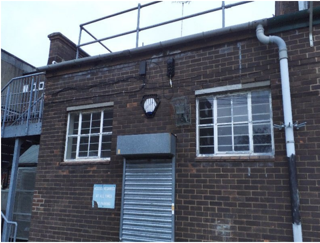
Sample No: 22/12/B/13/DAB12 External Below windowsill and frames Bitumen vapor barrier No Asbestos Detected
