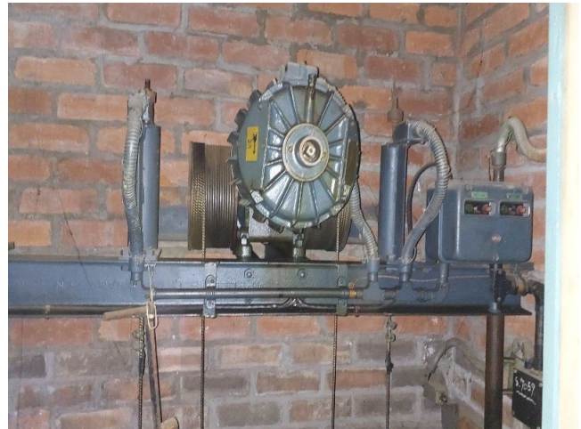
Sample No: No Sample 1.02 Lift Lift Brake pads containing: Chrysotile
