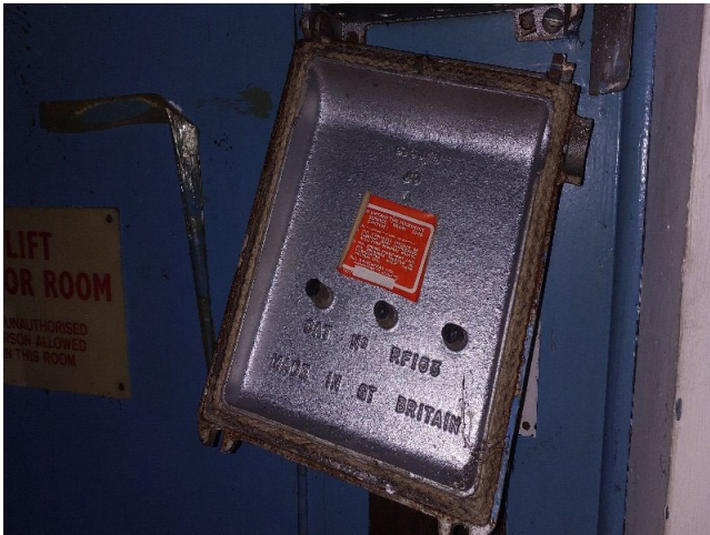
Sample No: Refer to Sample 22/12/B/13/DAB2 1.01 Stairwell Electrical fuse box Rope seal No Asbestos Detected
