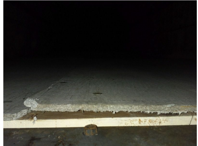
Sample No: 22/12/B/13/DAB6 G.08 Lift Internal Wall Asbestos Cement containing: Chrysotile
