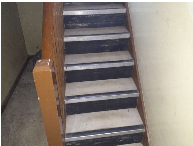
Sample No: Refer to Sample 22/12/B/13/DAB5 1.05 Stairwell Stairs Nose edging containing: Chrysotile
