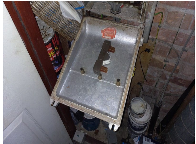
Sample No: 22/12/B/13/DAB2 G.03 Electrical cupboard Electrical fuse box Rope seal No Asbestos Detected
