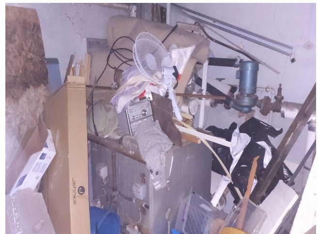
Sample No: No Sample 2.03 Boiler room Boiler and associated pipework Gaskets containing: Crocidolite
