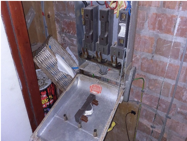
Sample No: 22/12/B/13/DAB1 G.03 Electrical cupboard Electrical fuse box Woven flash guards containing: Chrysotile
