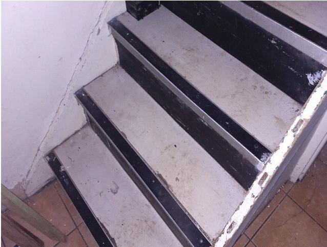
Sample No: 22/12/B/13/DAB5 G.07 Stairwell Stairs Nose edging containing: Chrysotile
