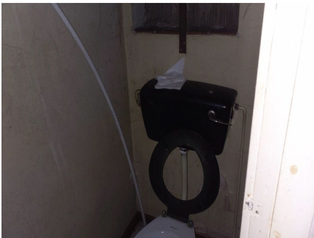
Sample No: 22/12/B/13/DAB11 2.05 Toilet Toilet cistern Thermoplastic containing: Amosite
