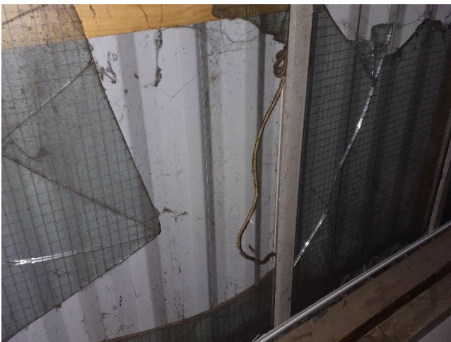
Sample No: 22/12/B/13/DAB7 1.01 Stairwell Windows Rope seal containing: Chrysotile
