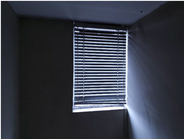
Sample No: Refer to Sample 22/12/B/13/DAB7 2.01 Landing Windows Rope seal containing: Chrysotile
