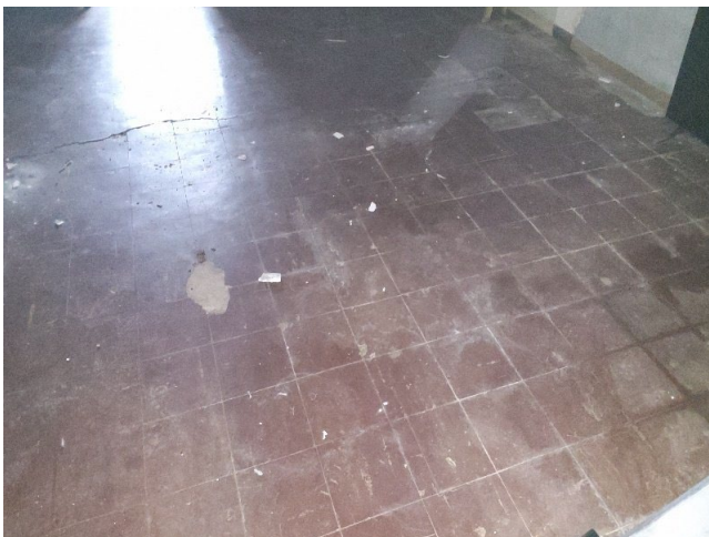
Sample No: 22/12/B/13/DAB8 1.03 Store room Floor Vinyl floor tiles containing: Chrysotile (In both tile and bitumen)
