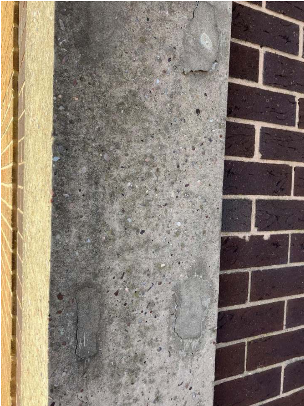
Local spalling to external concrete corner column at south east corner of store
