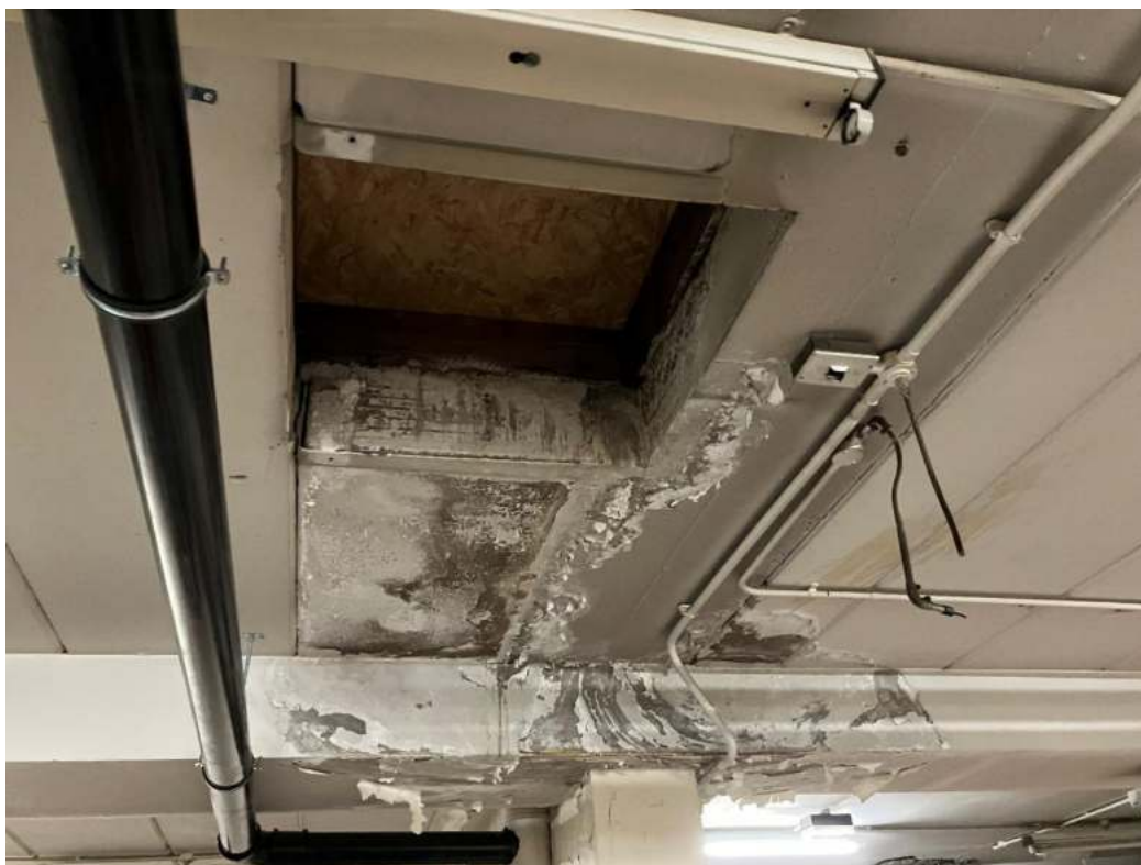
Boarded over opening through roof precast planks with evidence of water penetration
