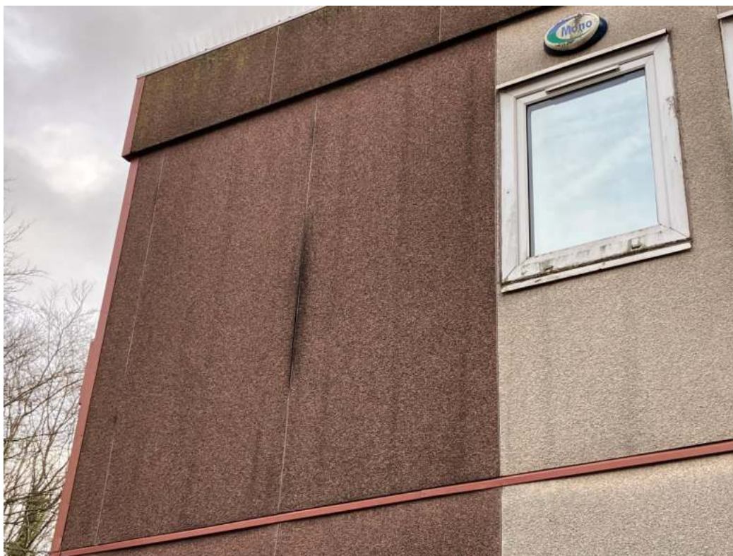
Separation of external cladding to first floor northern elevation of modular extension
