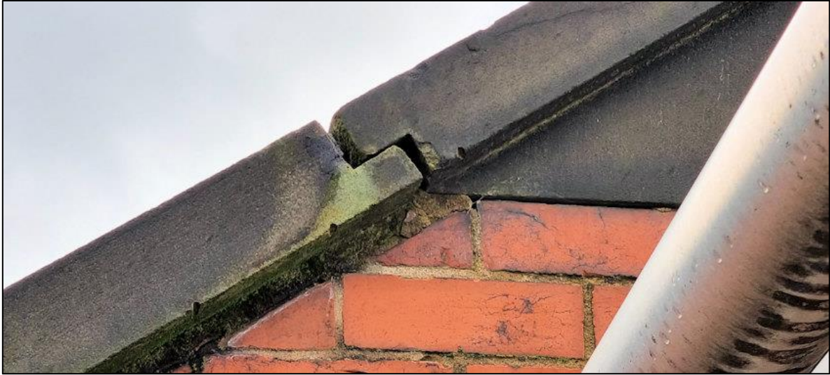
Plate 6: The gaps between the coping stones offered roosting potential.
