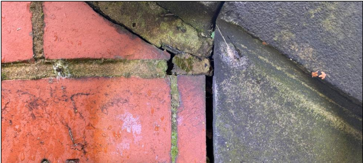
Plate 7: There were gaps noted at the junction between the walls and the end coping stones offering roosting potential.
