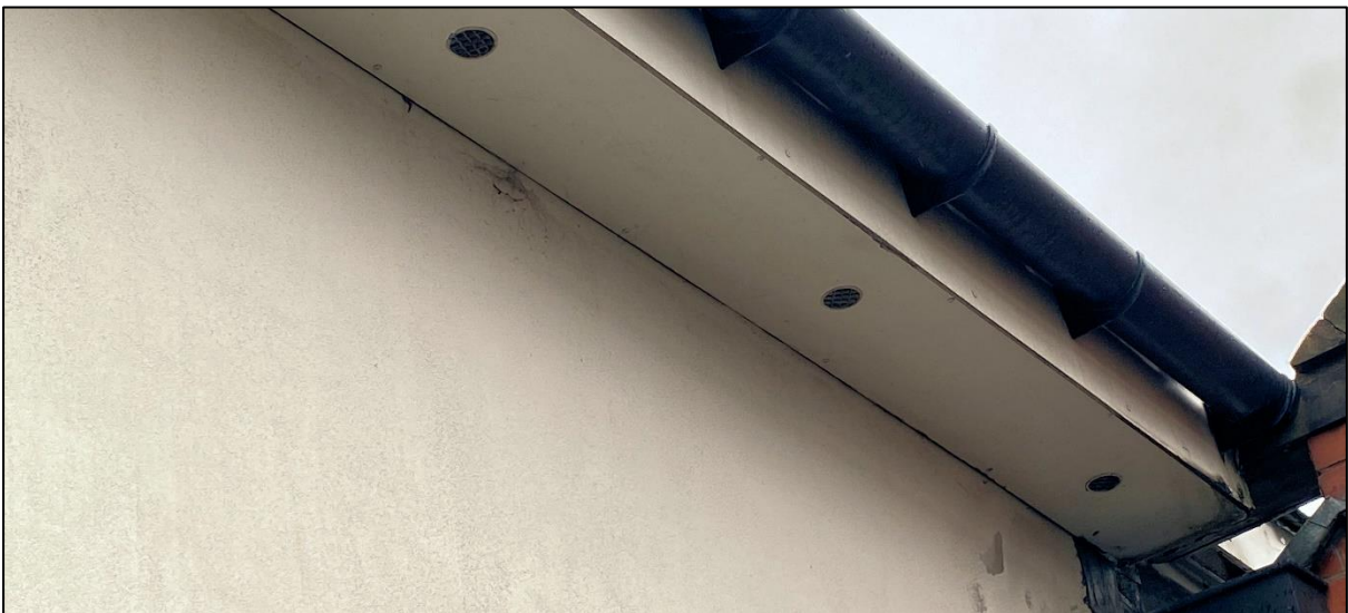
Plate 11: Soffits on the adjoining building were not well sealed and offered roosting potential.
