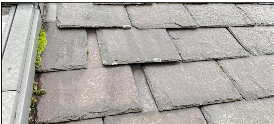
Plate 5: Gaps were noted beneath the flat tiles that offered further roosting opportunities.
