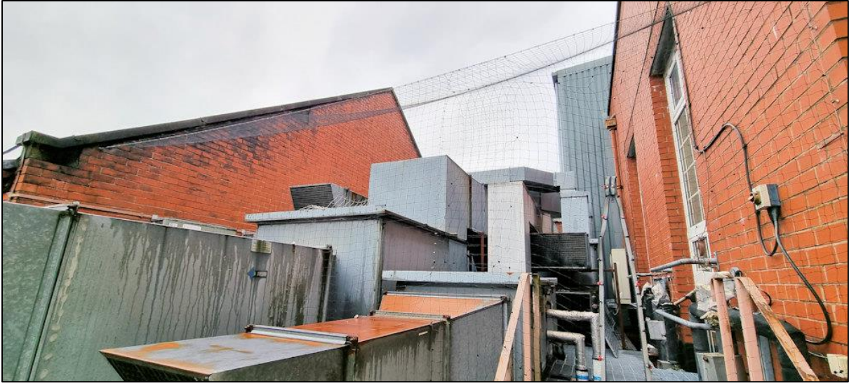
Plate 19: Bird netting around the external plant effectively excluded bats from some areas.
