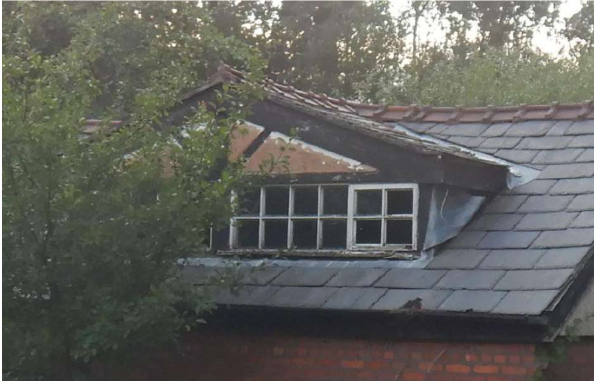
Photo 15. Southern aspect of the garage. Showing open windows and rot around window frame. A willow has since obstructed the western half of the dormer.
