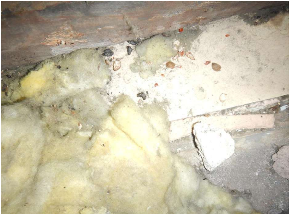
Photo 22. Rat droppings in eastern loft space.
