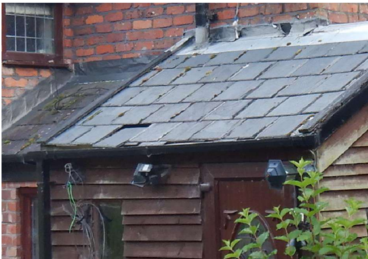
Photo 8. Lean-to on eastern aspect showing loose tile.
