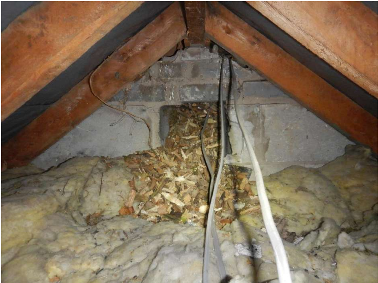
Photo 21. Showing northern gable of eastern loft space. More evidence of bird droppings and old nest.
