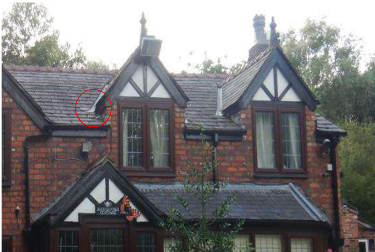
Photo 2. Gaps in tiles and loose flashing on the front of the house
