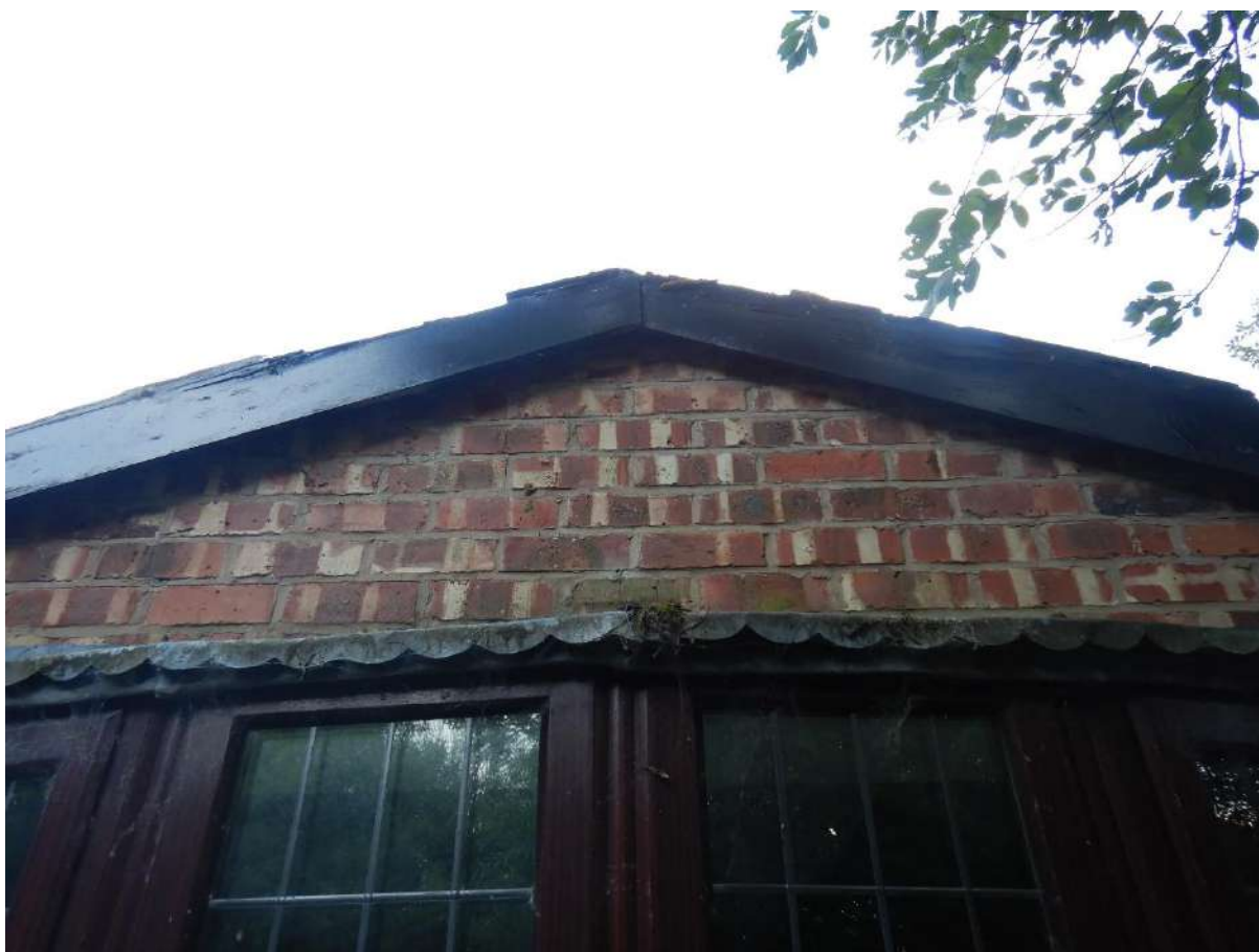
Photo 3. Gaps beneath the wooden fascia boarding.
