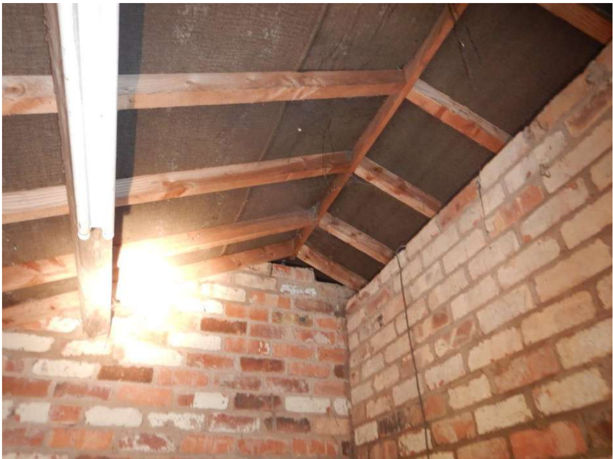
Photo 24. Log store internal showing gaps above the wall plate.
