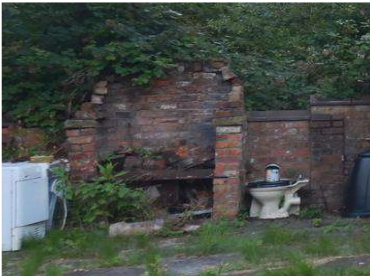
Photo 9. Brick BBQ in garden that has partially collapsed. Cracks in mortar provide PRFs for bats.
