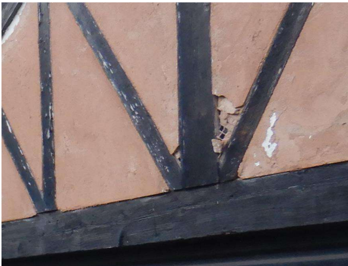
Photo 13. Showing damage to the gable rendering that was previously deemed superficial.
