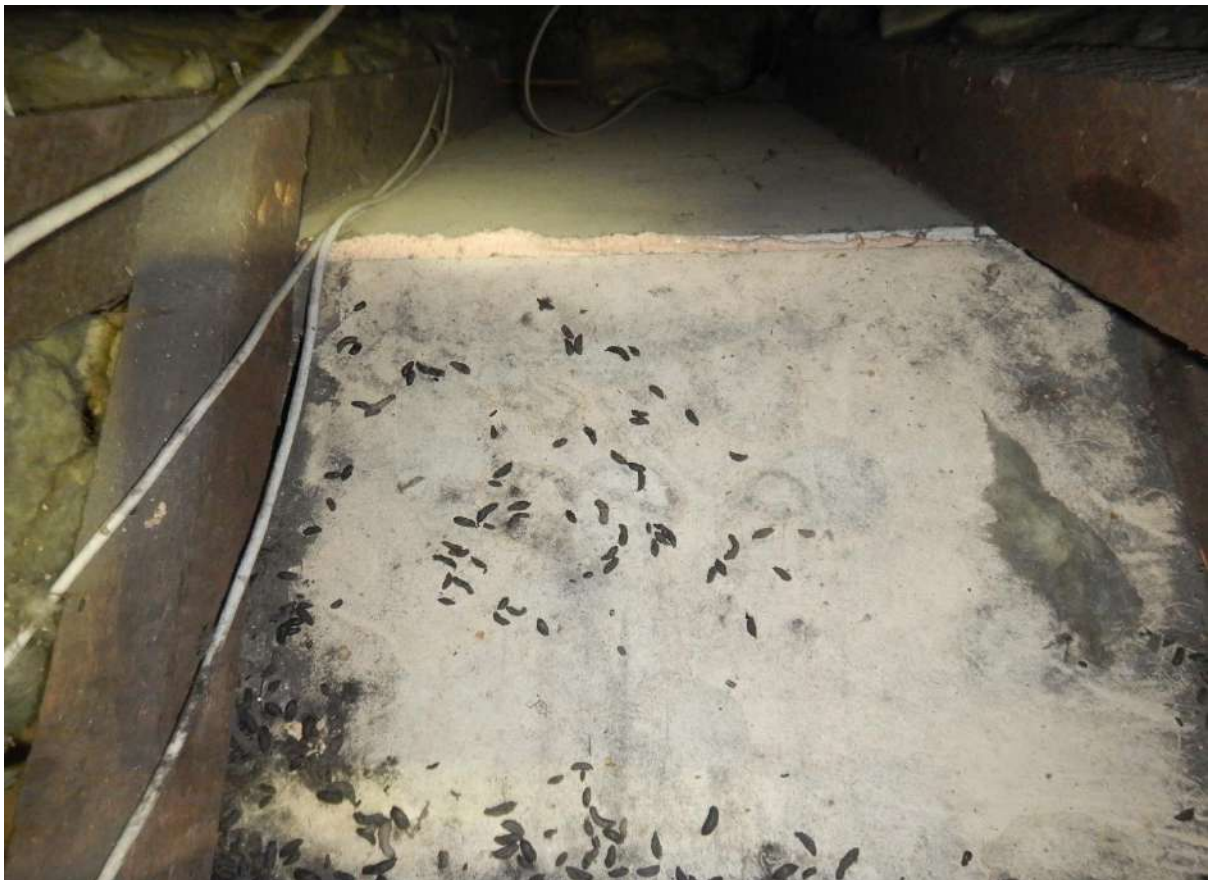
Photo 16. Mouse droppings in the loft space of the main house.
