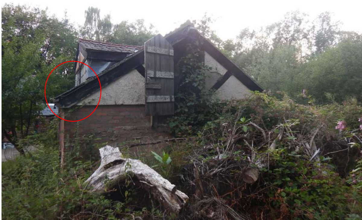
Photo 14. Rear of garage. Gaps between fascia and brick work, and broken verge pointing. Bramble has since encroached into the central door. Also showing damage to the verge pointing.
