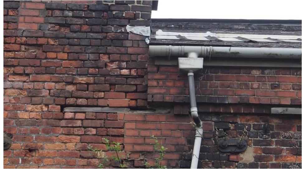
Inappropriate uPVC external rainwater goods in poor state of repair
