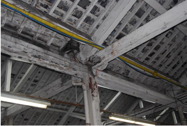
Deteriorating truss ends at valley gutter.
