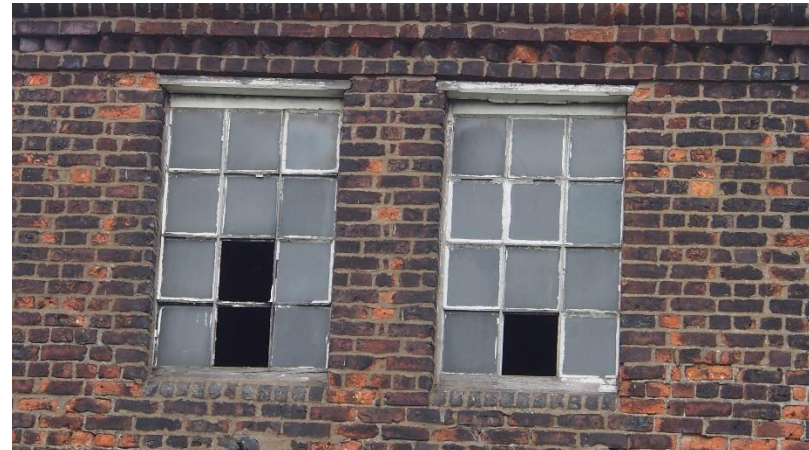
Original C19th window frames generally in poor condition and requiring major overalls.
