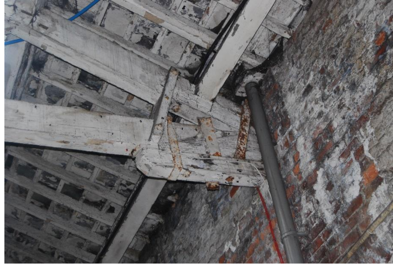
Poor quality 'historic' repair to truss ends.
