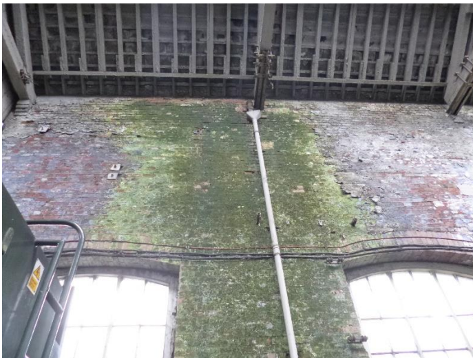
Long term problems of failed internal rainwater goods and water ingress.
