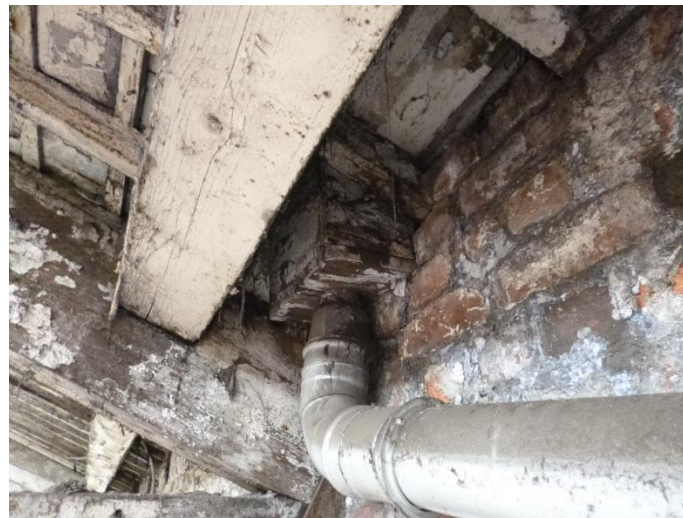
Failed internal hoppers causing issues for truss ends.
