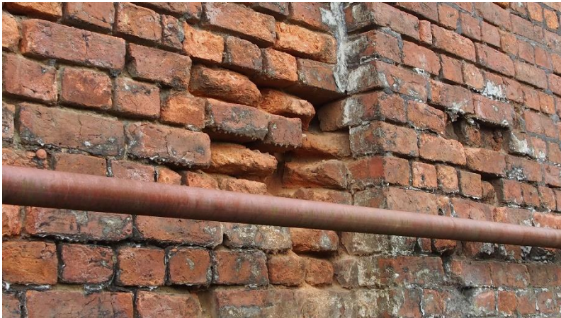
Areas of brickwork erosion – particularly to the west elevation.
