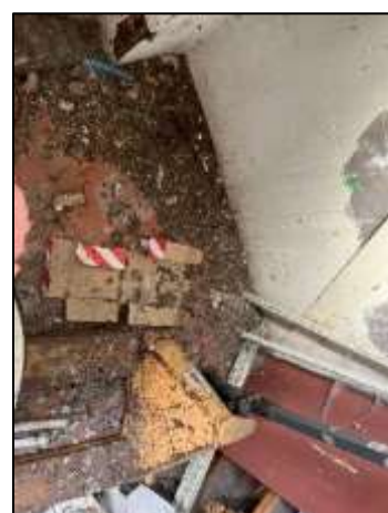
Bird droppings inside units 4
