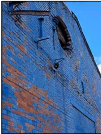
Hole in wall of east elevation
