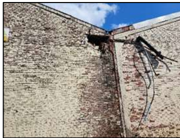
Hole in unit 8 west elevation wall
