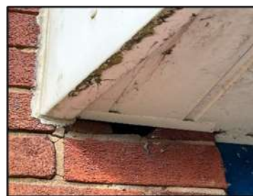
Gap between uPVC and the brick wall on the north elevation
