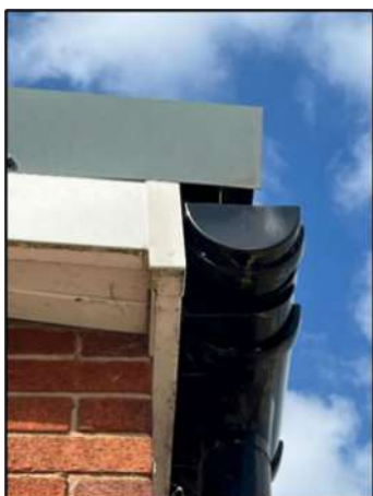
Gaps in the metal soffits on north elevation
