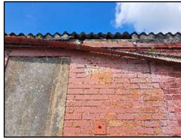
Gap under the roof on unit 8 south elevation
