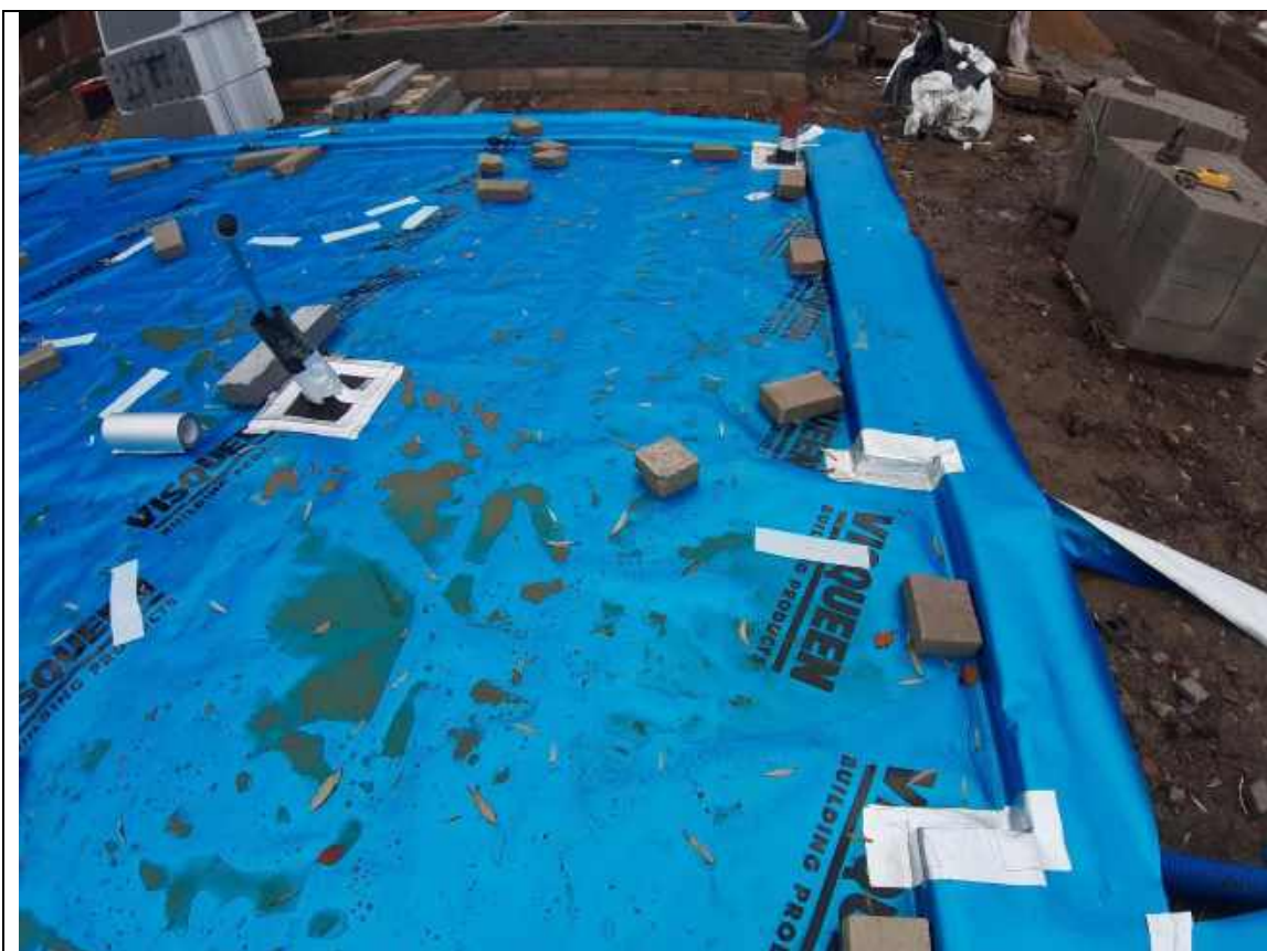
Plate 24: Showing the general condition of the membrane and sealed service entries on Plots 5&6
