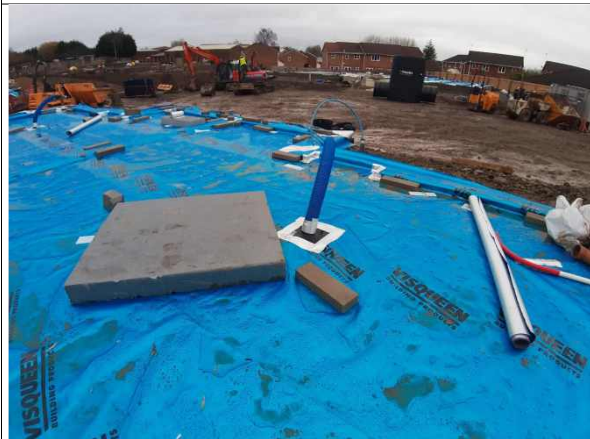
Plate 9: Showing the general condition of the membrane and sealed service entry on plots 3-4
