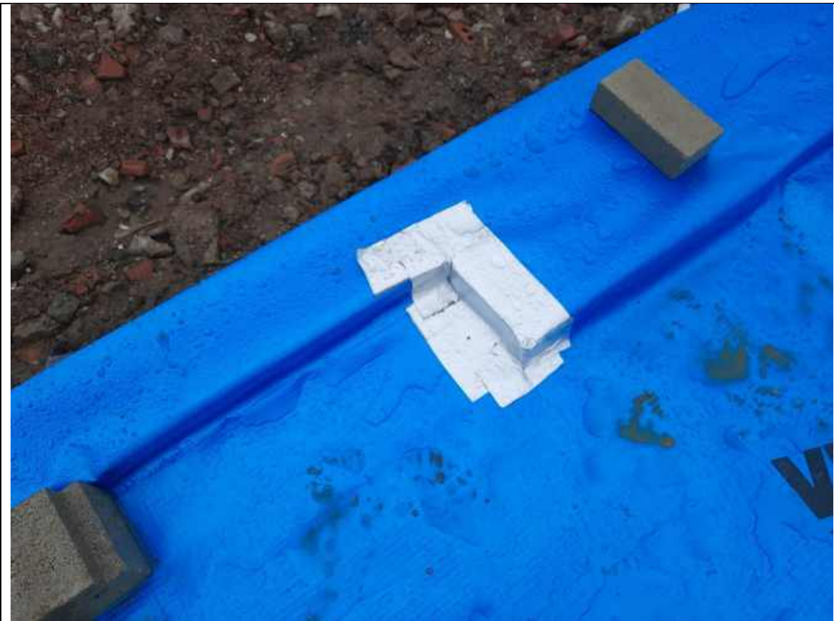
Plate 62: Showing the condition of the edges on Plot 19
