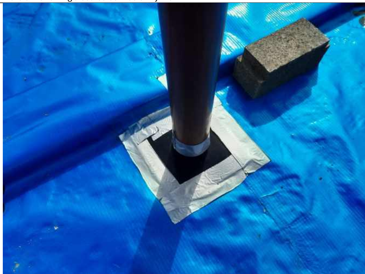
Plate 53: Showing sealed service entry on Plot 17
