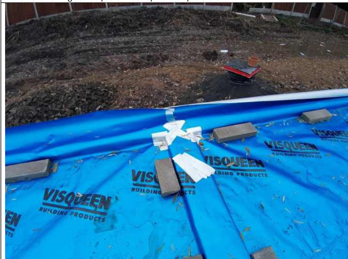
Plate 17: Showing the condition of the membrane sealing on plots 5-6
