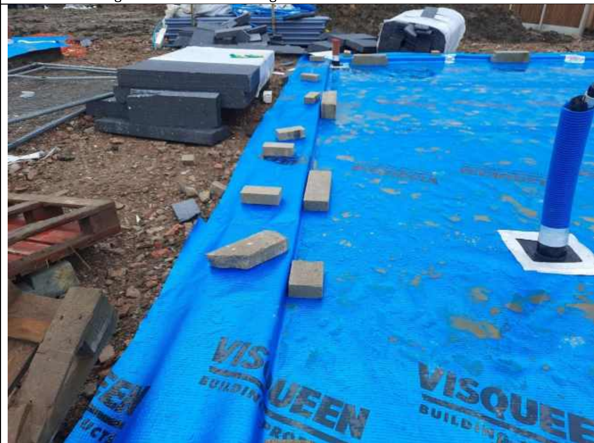
Plate 61: Showing the condition of the edges on Plot 19
