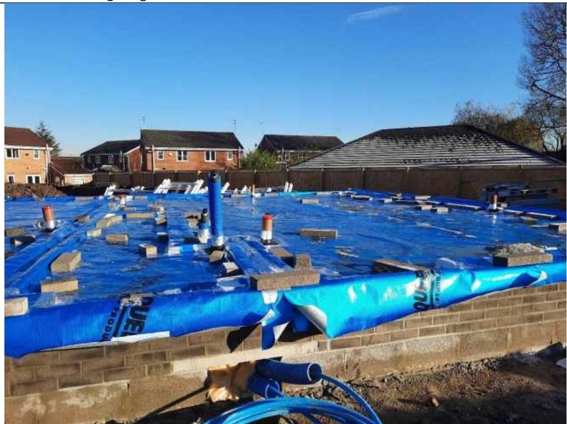
Plate 81: Showing the general condition of the membrane and sealed service entries and preformed top hats in Plots 25-26
