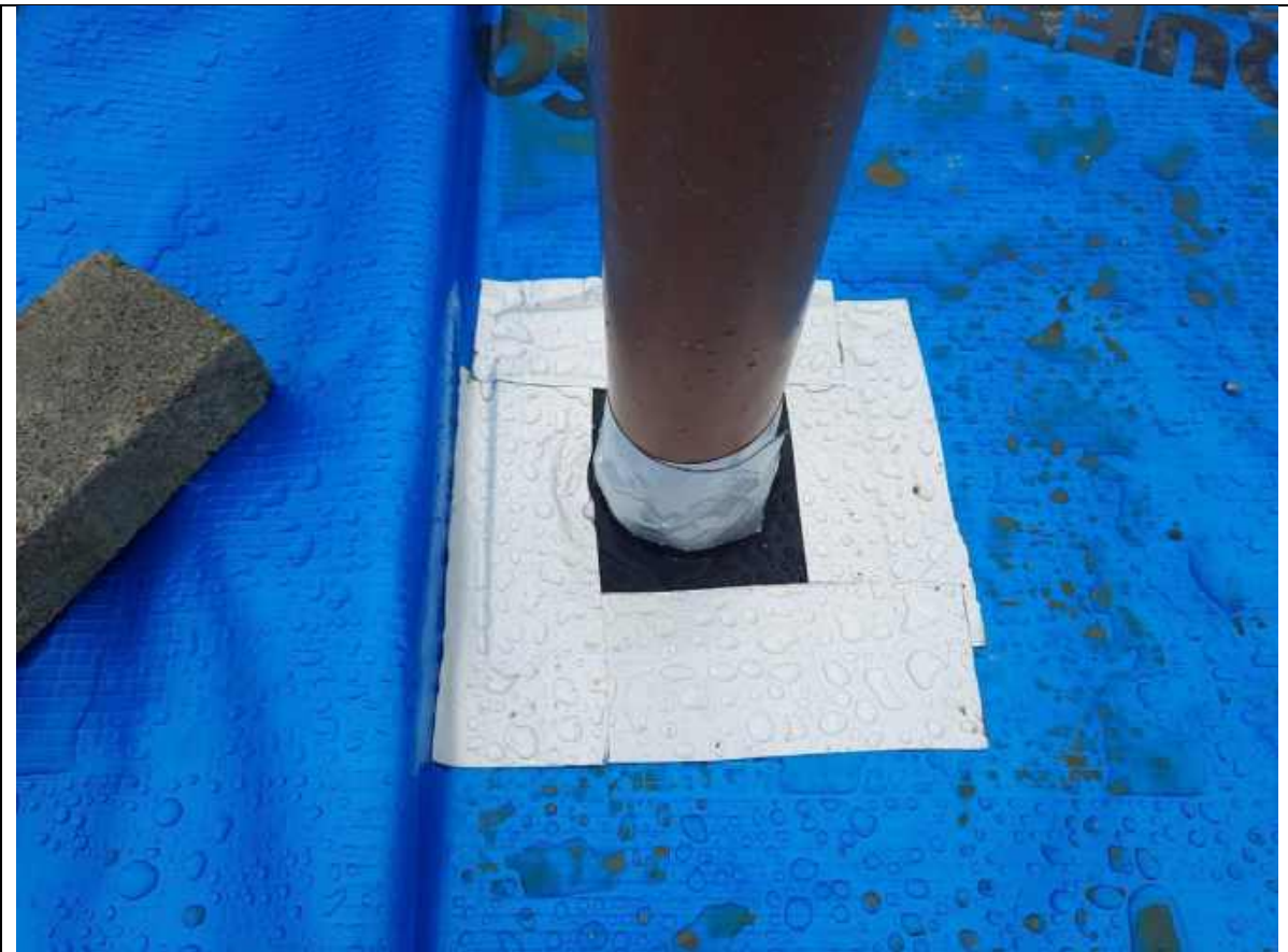
Plate 60: Showing the condition of the edges on Plot 19
