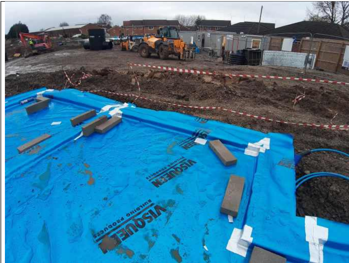
Plate 4: Showing the general condition of the gas membrane on plots 1-2
