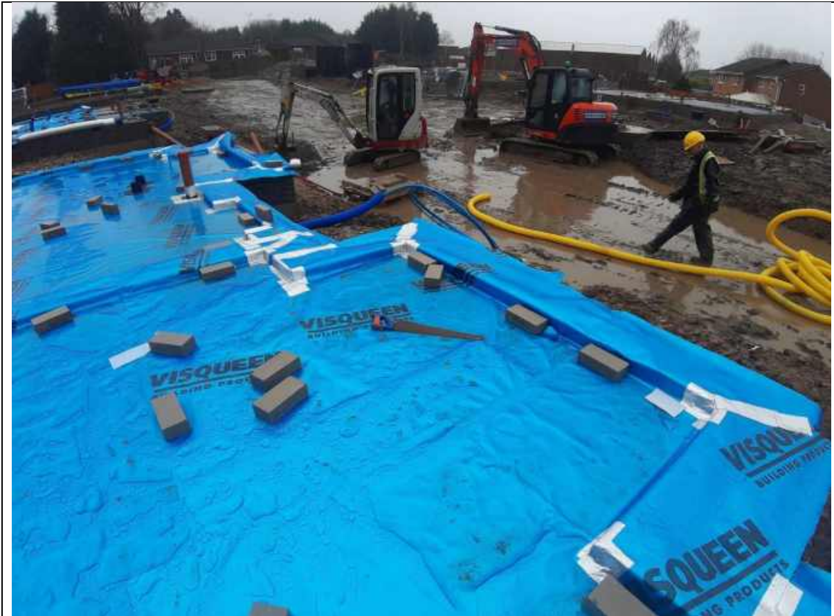
Plate 34: Showing the condition of the membrane on Plots 9-10
