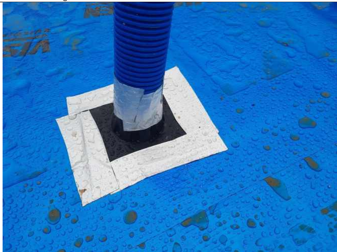
Plate 65: Showing a sealed service entry on Plot 20
