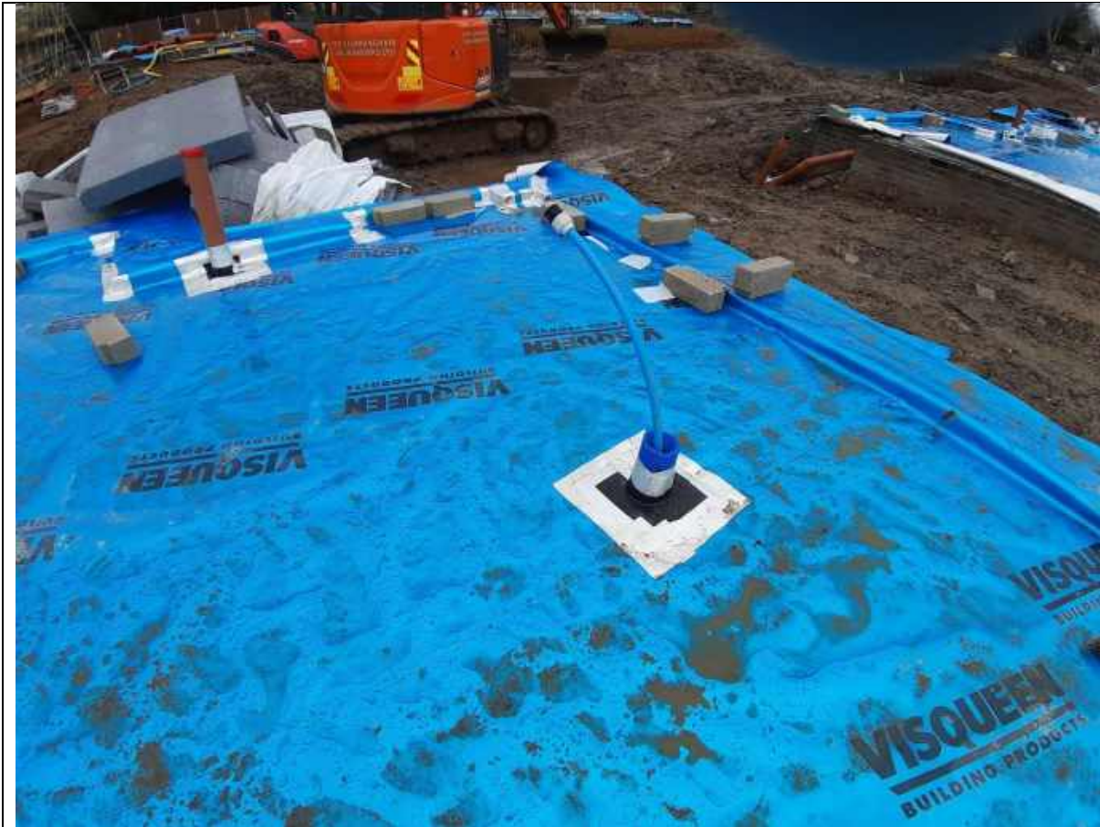
Plate 75: Showing a sealed service entry on Plots 23-24
