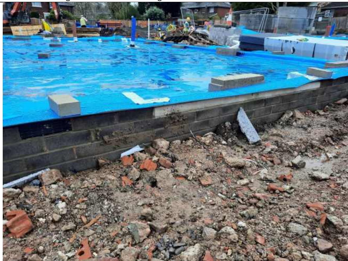
Plate 63: Showing the condition of the membrane on Plot 19
