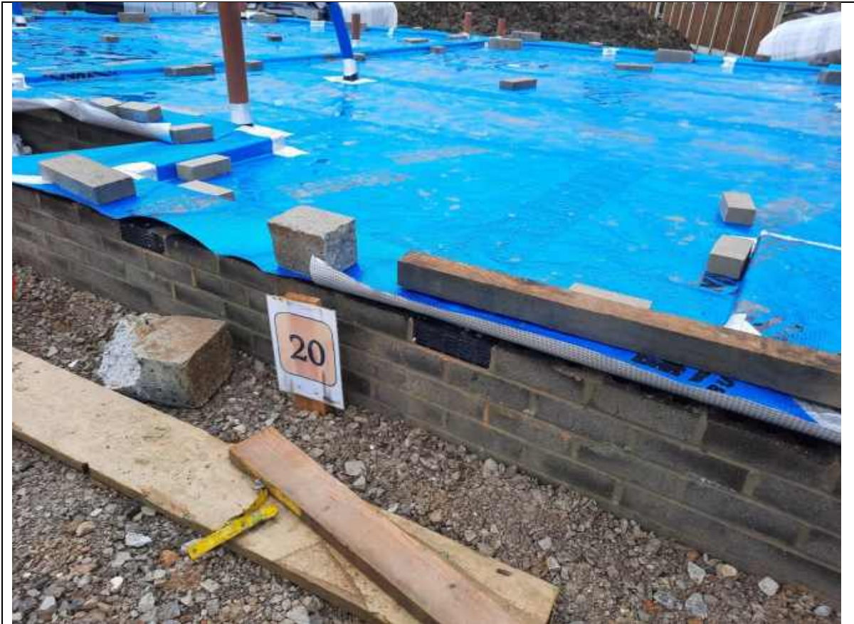
Plate 66: Showing the condition of the membrane on Plot 20
