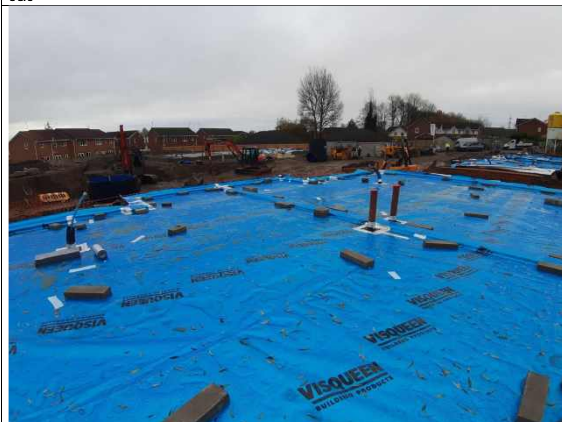
Plate 25: Showing the general condition of the membrane and sealed service entries on Plots 5&6
