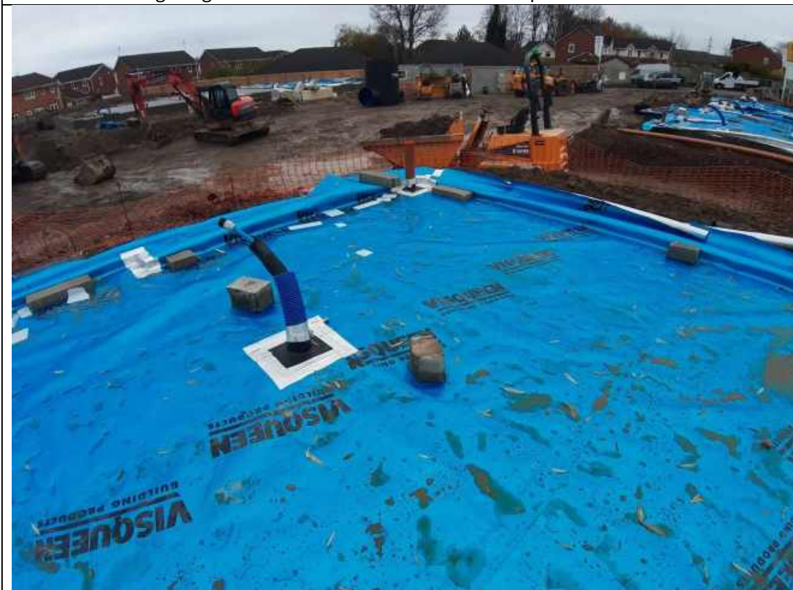
Plate 21: Plots 5&6: Showing the general condition of the membrane and a sealed service entry on plots 5&6
