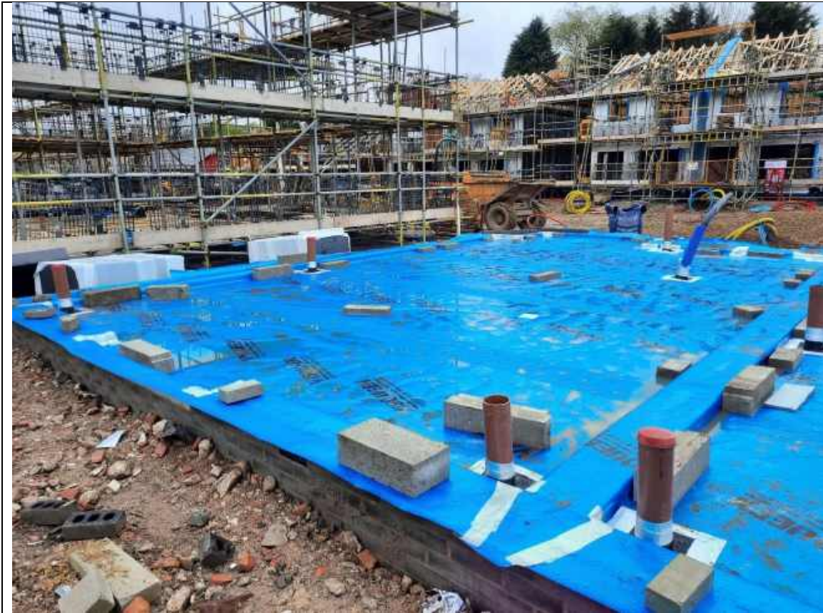
Plate 64: Showing the condition of the membrane on Plot 20
