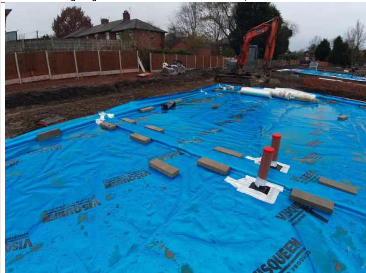
Plate 11: Showing the general condition of the membrane and sealed top hats on plots 3-4
