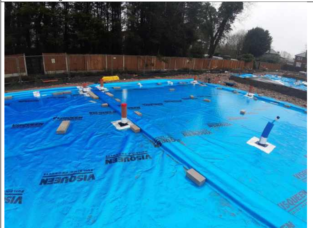
Plate 35: Showing the condition of the membrane Plots 9-10
