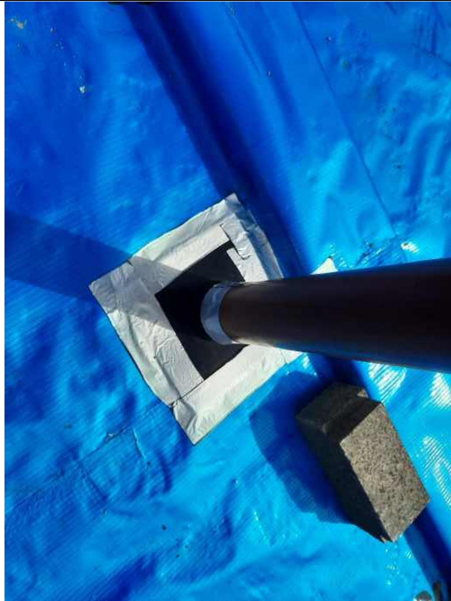
Plate 49: Showing a sealed service entry on Plot 16
