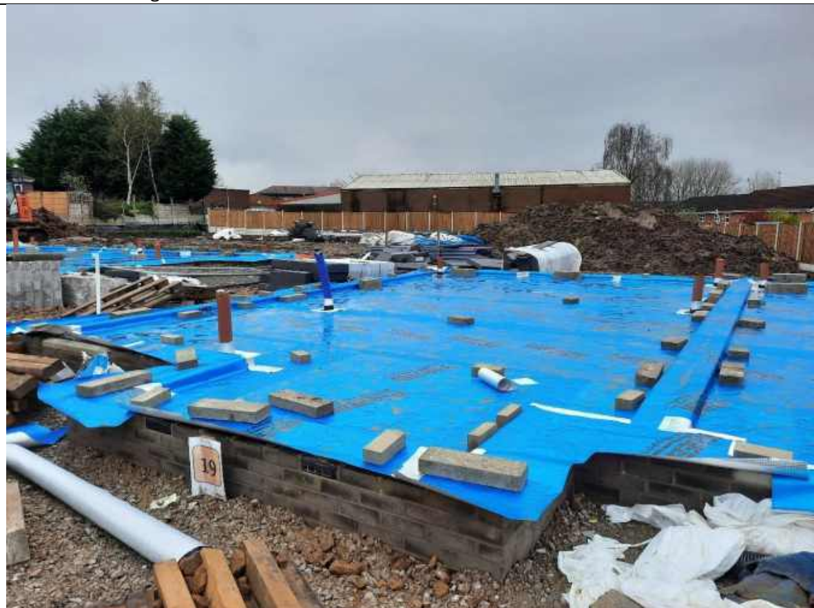
Plate 59: Shwoing the general condition of the membrane on Plot 19
