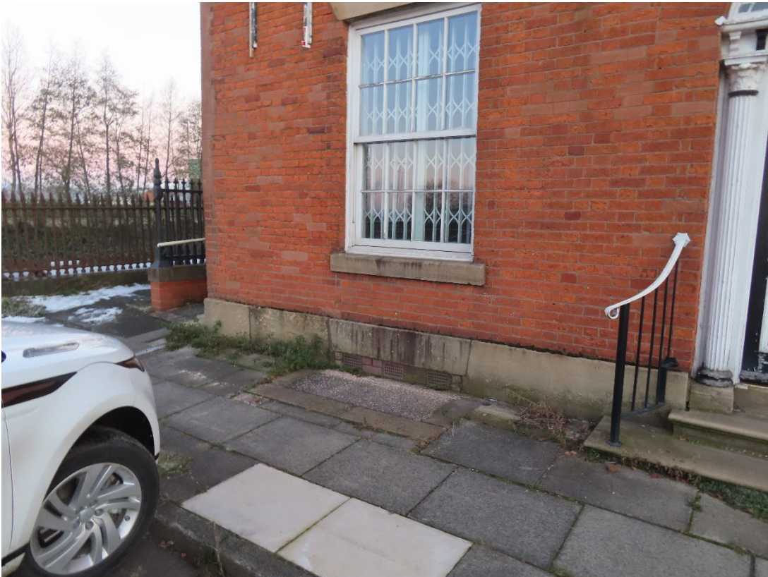
Previous brick repairs to front wall of number 20.
