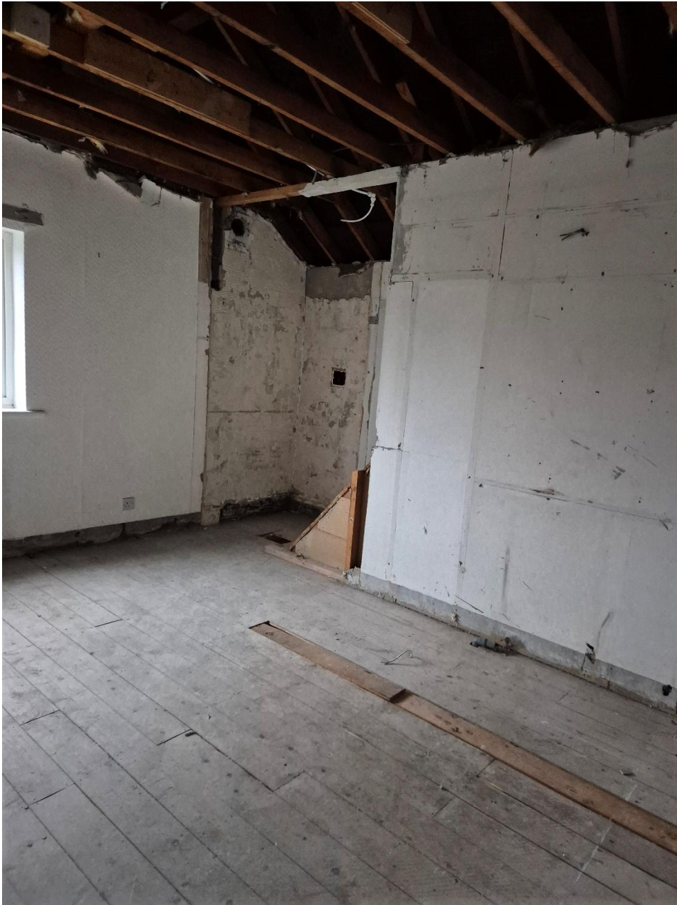
Photograph 3: Internal structure showing exposed plaster board and timbers.
