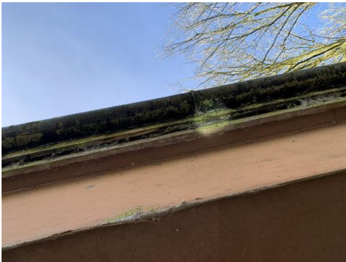
Plate 11 – Slight gap behind the fascia on same section of building, discounted from recent use due to the heavy cobwebbing
