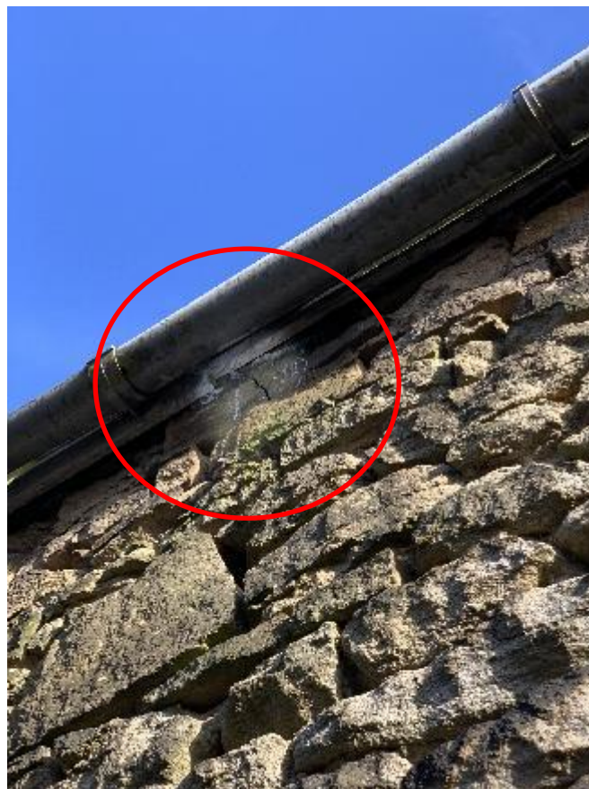
Plate 5 – Evidence of birds using the gap at wall plate level, with droppings visible
