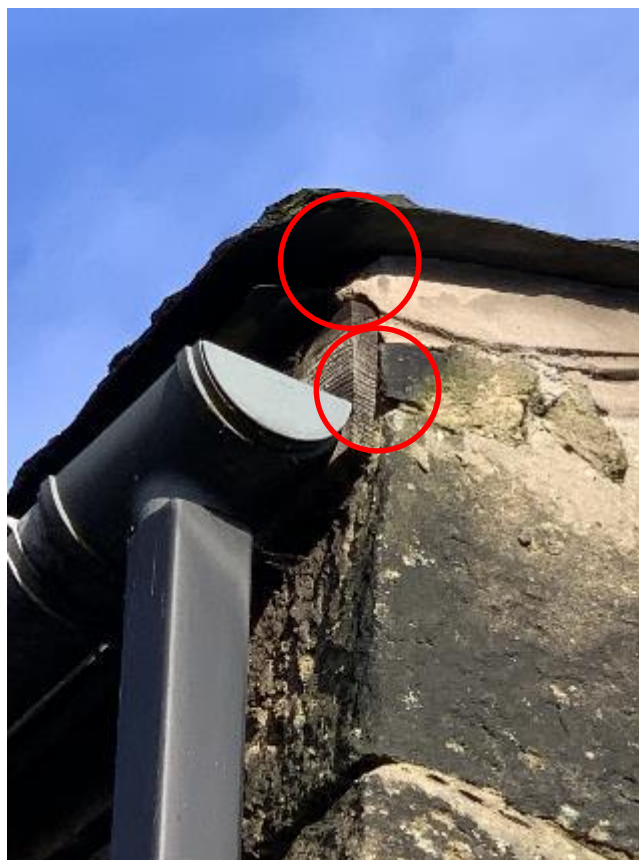
Plate 2 – Potential ingress point behind fascia and below roof slate
