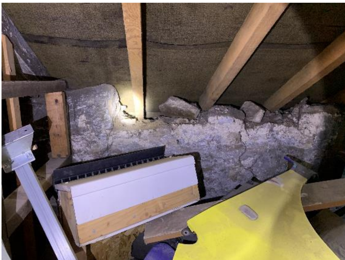
Plate 19 – Clear evidence of gaps at wall plate level
