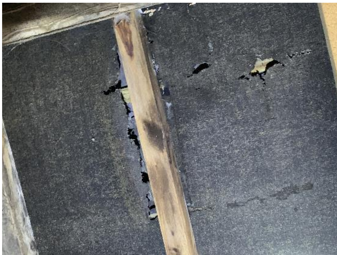
Plate 18 – Poor state of repair of bitumen 1F underfelt
