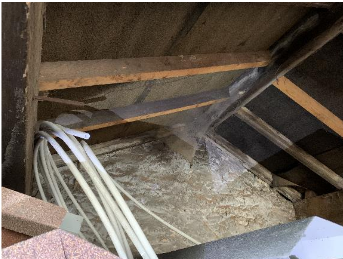
Plate 17 – Presence of bitumen 1F underfelt evidenced, with heavy cobwebbing in some parts
