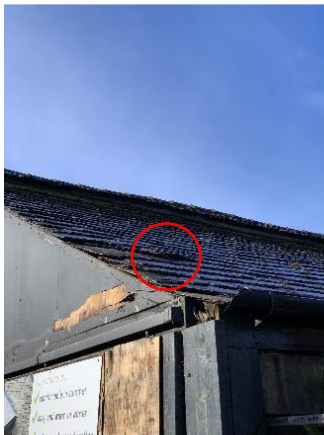
Plate 7 – Poor state of slate roof providing ingress opportunities
