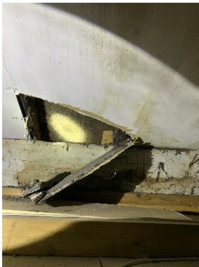
Plate 9 – Evidence of bitumen 1F underfelt behind boarding in same loft space
