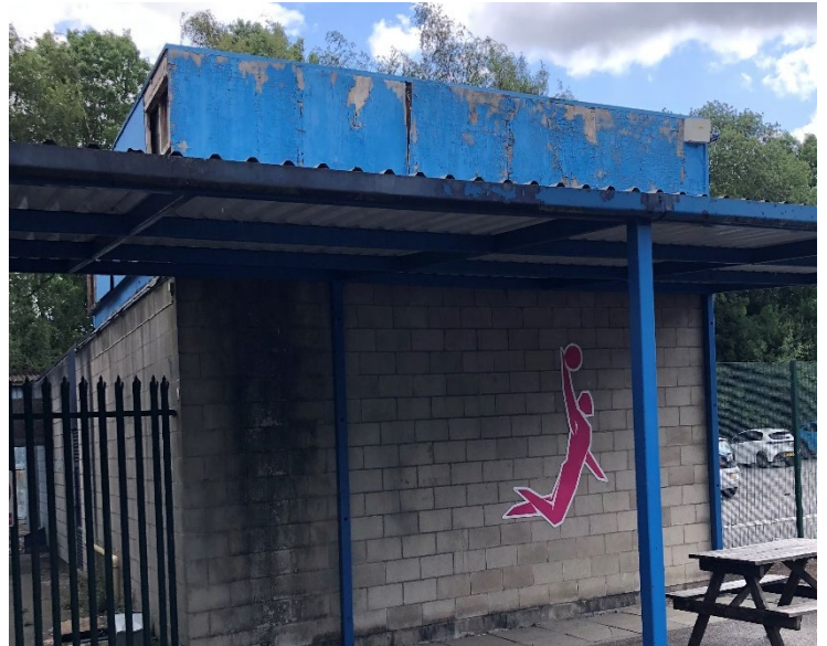
Figure 8: Western side of leisure centre entrance detailing building with wooding cladding containing numerous gaps and potential roost features.
