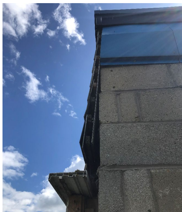
Figure 6: Gaps between brick, timber cladding, hung slates and fascias on south-west elevation of school building adjacent to playground area.
