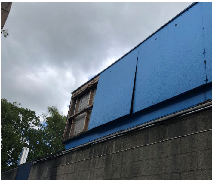
Figure 9: Same building, image taken from northern elevation.
