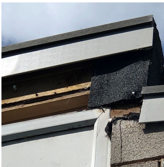
Figure 5: Missing cladding. gaps in fascia boards and felting between soffit and brickwork on southern elevation of school building in front of MUGGA area.
