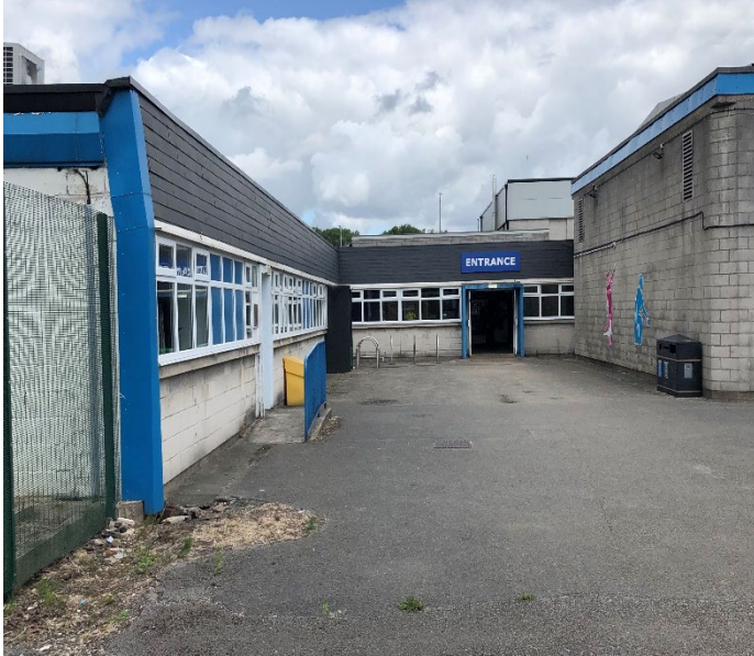
Figure 7: Entrance to leisure centre detailing extensive slate cladding with gaps, and fascias in poor condition with gaps between roofing materials and brickwork.
