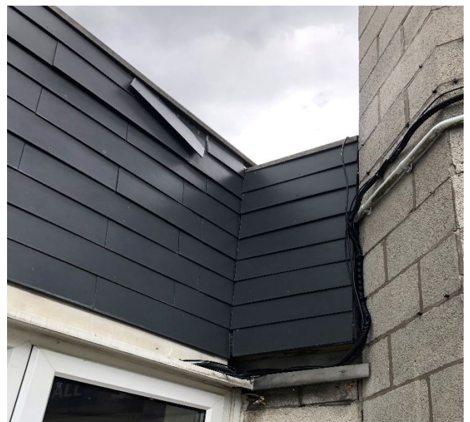
Figure 10: South-east elevation of leisure centre entrance with damaged fascias and cladding containing PRF's
