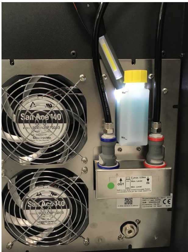
Figure 83: Checking the cooling liquid level
