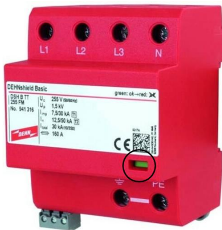
Figure 80: Check of overvoltage protection
