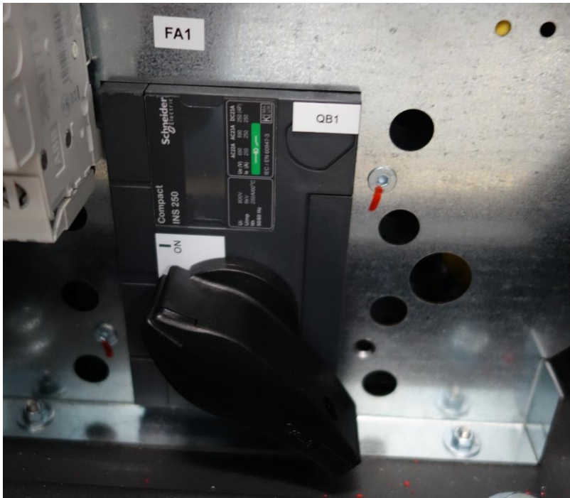
Figure 78: Function test of main switch
