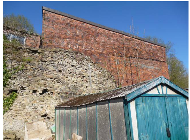
Eastern elevation with multiple gaps / holes between brickwork and within dilapidated stone wall.
