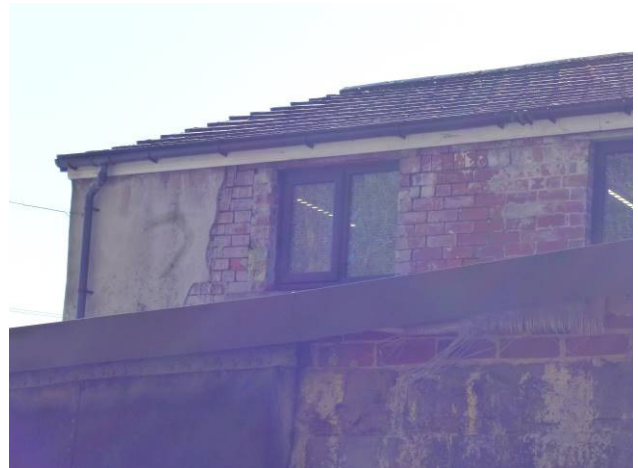
Western elevation viewed from Paradise Street. Significant gaps between brick courses and behind damaged render.
