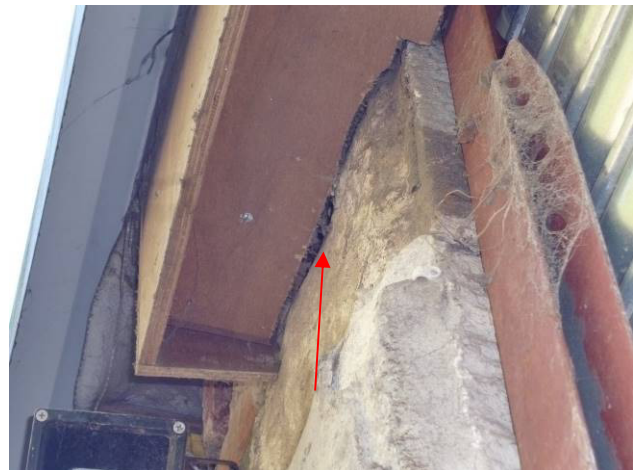
Western elevation, Paradise Street. Gaps between stone and soffit.
