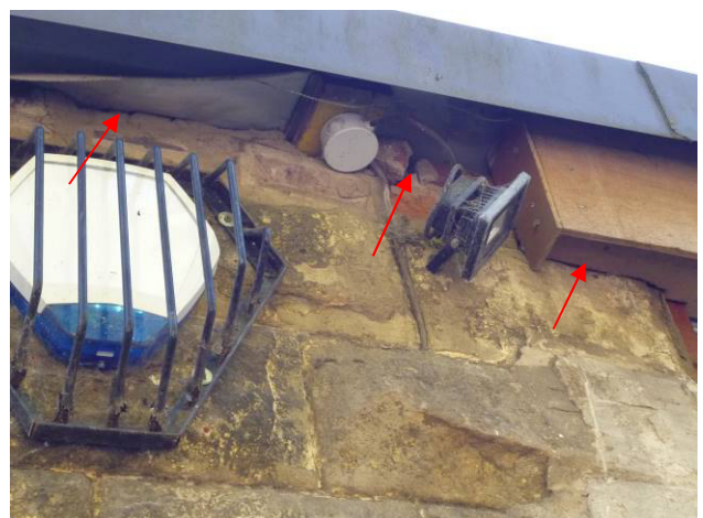
Western elevation, Paradise Street. Gaps between stone and soffit and roof overhang.
