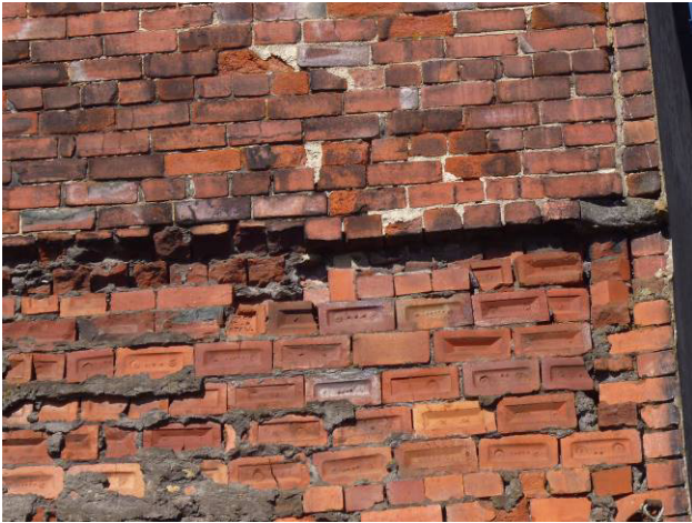
Eastern elevation with multiple gaps / holes between brickwork.
