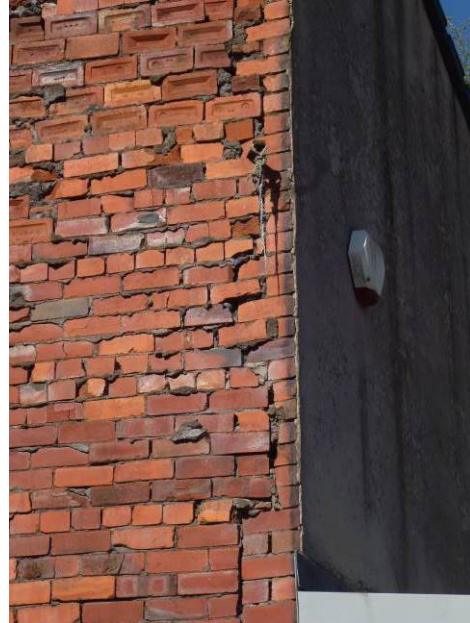
Eastern elevation with multiple gaps / holes between brickwork.
