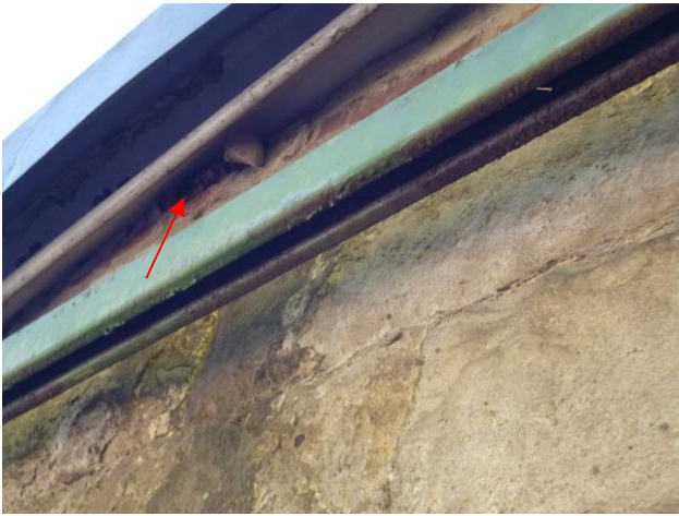
Western elevation, Paradise Street. Gaps between stone and fascia.
