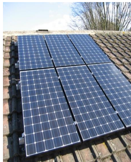
Figure 8 - Photovoltaic array on a pitched roof
