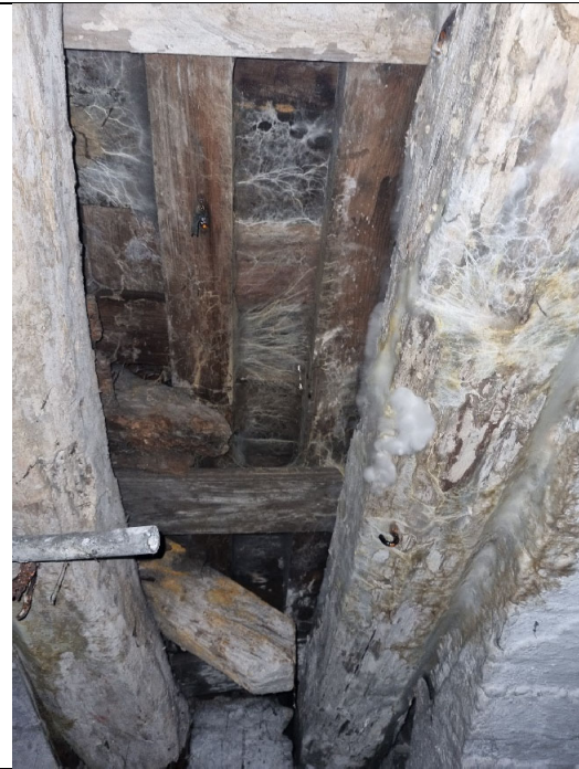
PHOTOGRAPH 10 (Above) – Extensive and active dry timber rot infestation.
