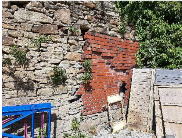
Figure 7 - Looking north; the northern site boundary is a retaining wall which appears to be in poor condition.
