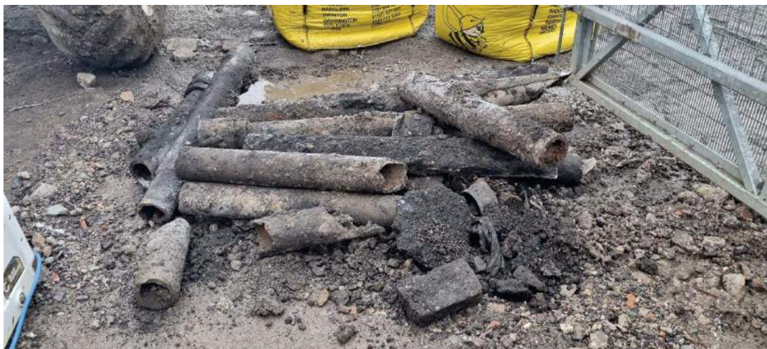
Figure 39 : 17/01/23 – Quarantine of asbestos-cement pipes encountered during final turnover
