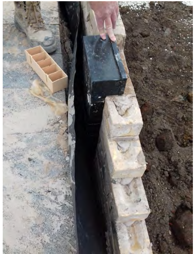
Photograph 8: Showing a periscopic vent which was installed on Plots 28-31 during inspection on 7 th April 2017.
