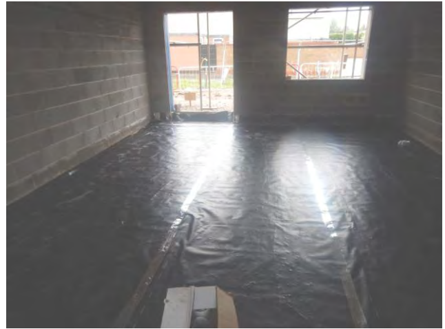
Photograph 14: Showing the general condition of the membrane installation on Plot 9 during inspection on 27 th July 2017.
