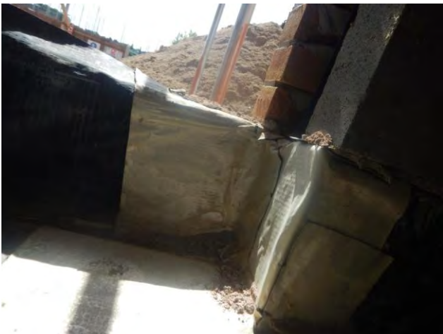
Photograph 23: Showing the membrane jointed to the perimeter stage one membrane underneath the blockwork and formation around the corner and door threshold using detailing strip with >150mm overlap and the condition of the corners on Plot 4 during inspection on 14 th August 2017.
