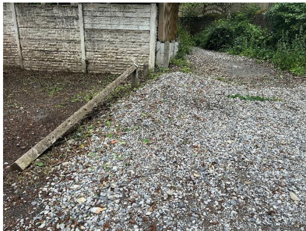
Damaged timber rail and washed stone
