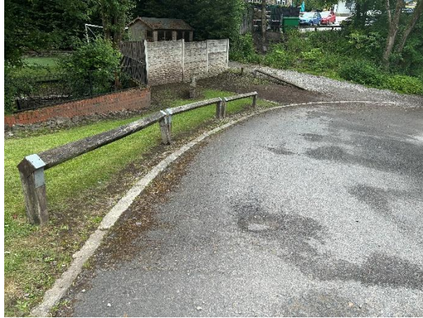
Start of another smaller pothole outside No 2
