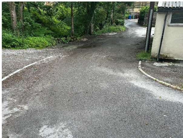
Road condition poor next to telegraph pole
