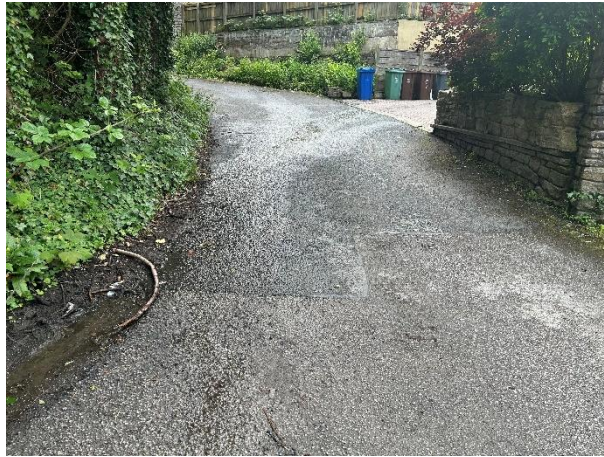
Road exit to Hare and Hounds, but shows a joint line for a recent tarmac reinstatement
