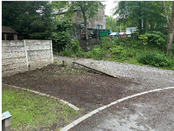
Damaged timber knee rail adj bridleway
