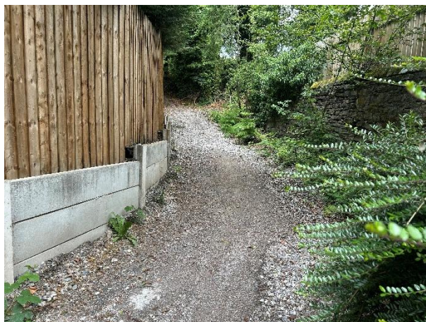
Poor condition to bridleway where stone washed away
