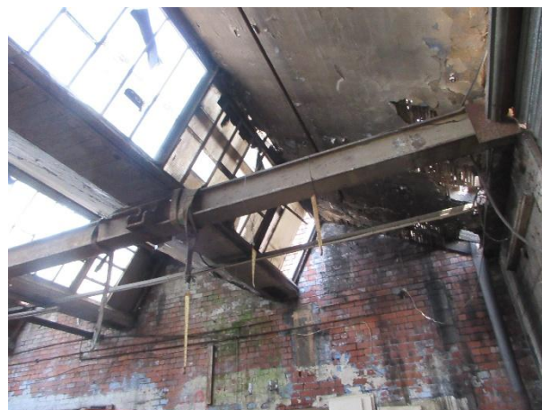
Photo 6: Example of conditions inside B1 showing frequent damage to roof and exposed conditions
