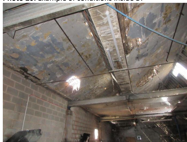
Photo 22: Example of conditions inside B7
