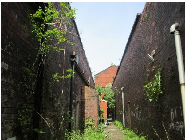
Photo 19: Gap between sections of B7
