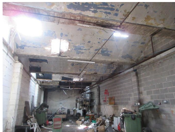
Photo 20: Example of conditions inside B7
