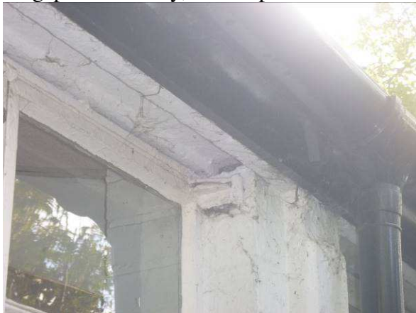
P5 Crevice above window frame, north aspect
