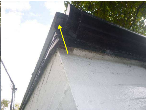
P2 Close-up of gap, similar gaps at all corners
