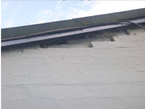
P3 gaps in masonry, west aspect
