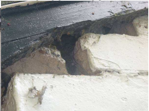
P4 Close-up of gap, similar gaps in both buildings
