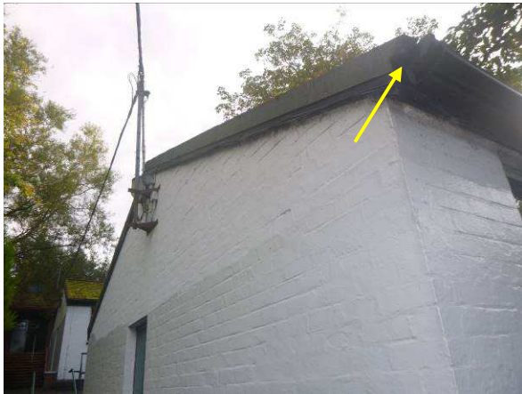
P1 Gable at west aspect, gap at corner
