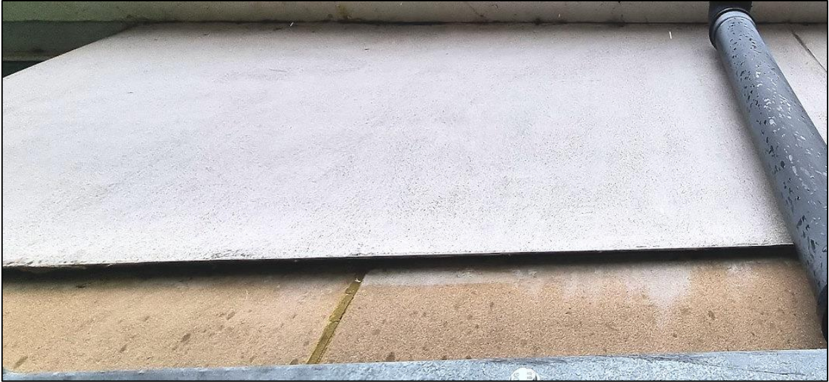
Plate 12: Cladding on the adjacent building was also found to have gaps beneath offering roosting potential.
