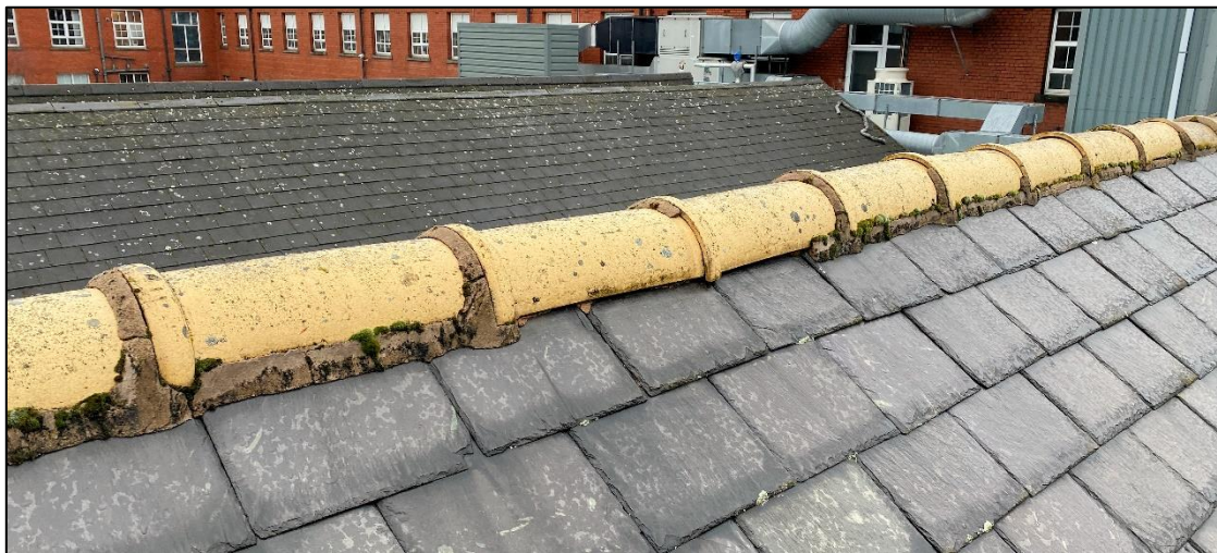
Plate 4: Whilst the roof was intact, gaps beneath the ridge tiles offered roosting opportunities.
