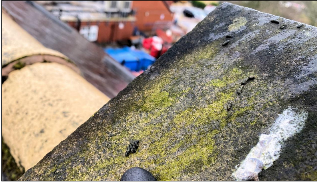
Plate 17: Droppings were noted on the coping stones but were not confirmed as bat droppings.
