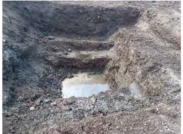
11.06.25 – Water ingress into well investigation trial pit
