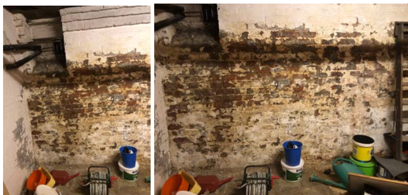
Image 04: existing water egress damage (in basement area)
