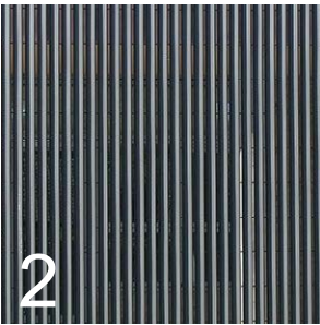
Metallic louvred plant screen
