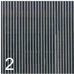
Metallic louvred plant screen
