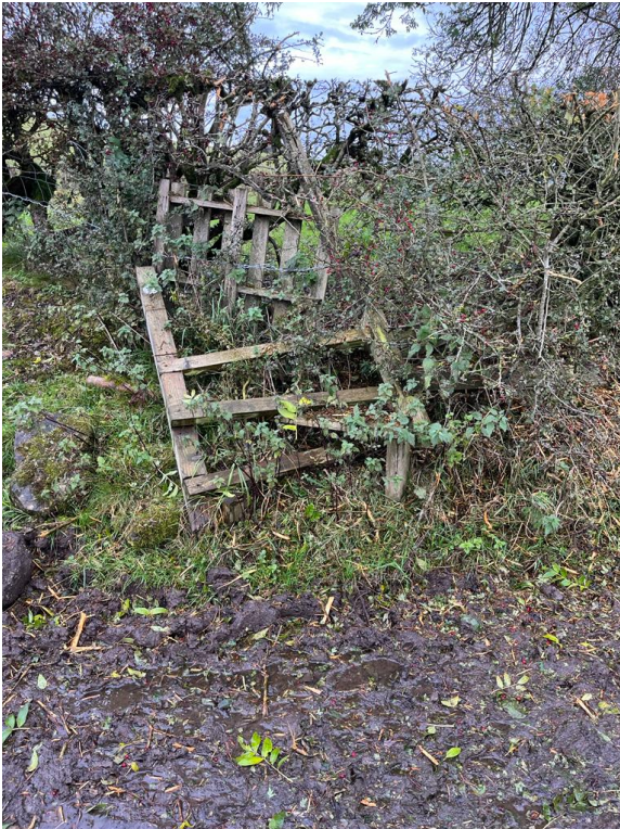
Damaged stile at intersection of PRow No.136 and PRow No. 138
