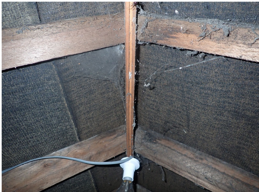
8 – Roof timbers are covered with dusty cobwebs.
