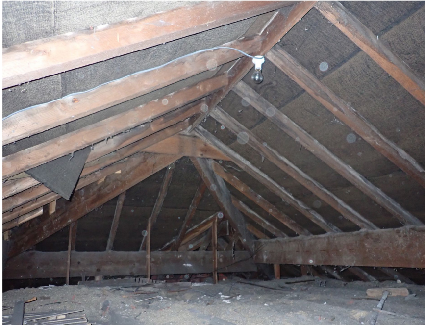
7 – No gaps in felt and eaves in pitched roof void and was not being used for storage.
