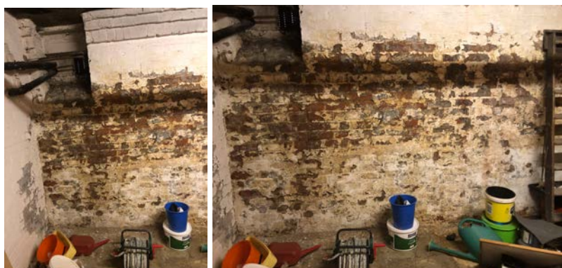
Image 04: existing water egress damage (in basement area)
