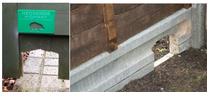
Insert 5: Showing wildlife access gap within fencing
