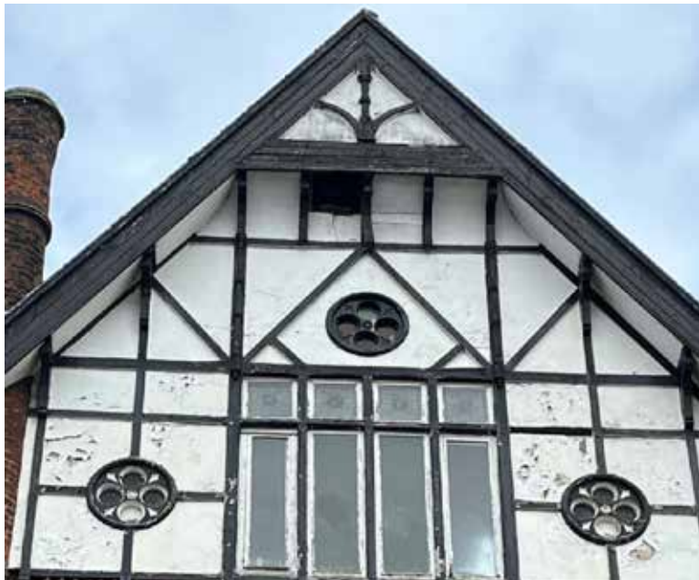
Image: Evidence of former roof light location- with one pane remaining glazed. Image: Deteriorating front elevation with timber and plaster.
