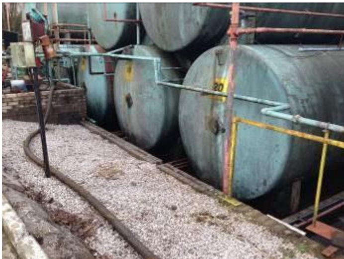
Plate 8 – Solvent Storage Tanks in Farm Northern Sector
