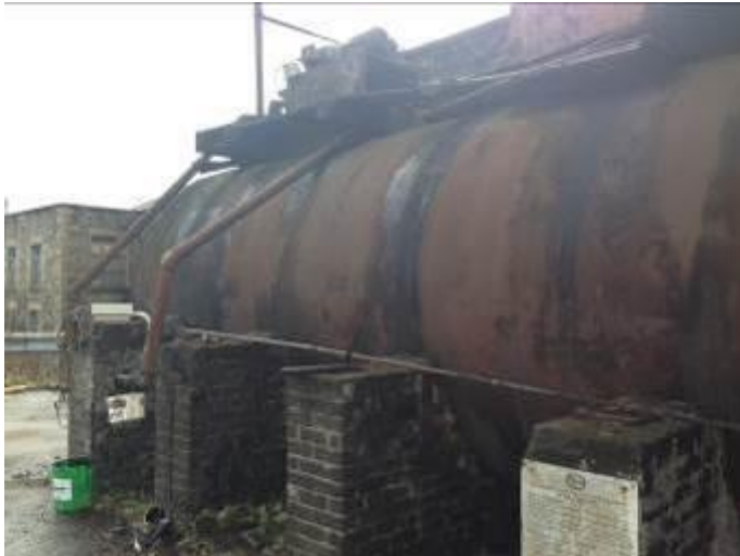
Plate 4 – Bitumen Tank on Reservoir Dam
