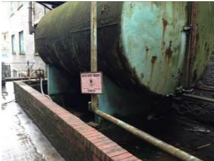
Plate 10 - Solvent Storage Tanks in Central Sector
