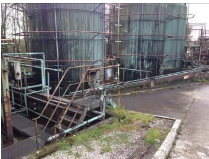
Plate 9 - Large Solvent Storage Tanks in Northern Tank Farm
