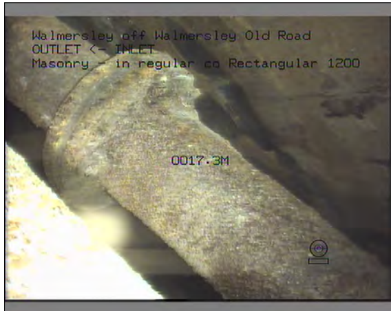
Photo: 013.JPG 17.3m, General remark
