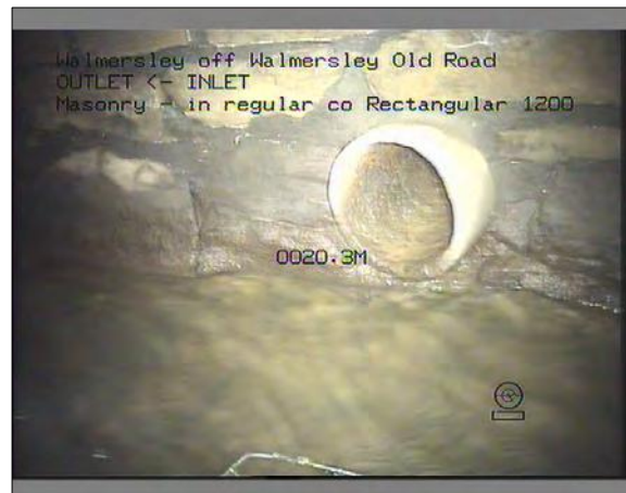
Photo: 016.JPG 20.3m, Connection intruding, at 5 o'clock, diameter 150mm, intrusion 05%
