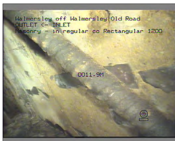
Photo: 008.JPG 11.9m, General remark
