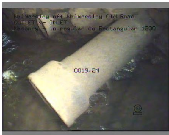
Photo: 015.JPG 19.2m, Connection intruding, at 5 o'clock, diameter 150mm, intrusion 20%
