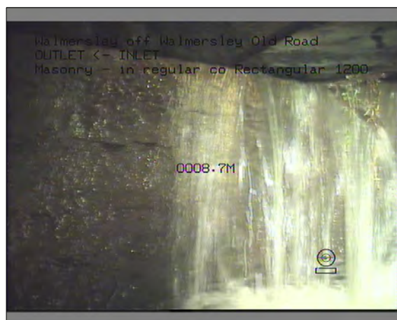
Photo: 006.JPG 8.7m, General remark
