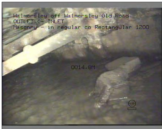
Photo: 011.JPG 14.8m, Settled deposits, other, 20% cross-sectional area loss
