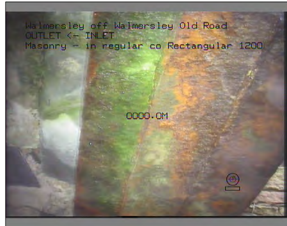
Photo: 002.JPG 0m, General remark
