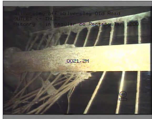
Photo: 018.JPG 21.2m, Other obstacles, other object in invert, from 1 to 6 o'clock, 85% cross-sectional area loss
