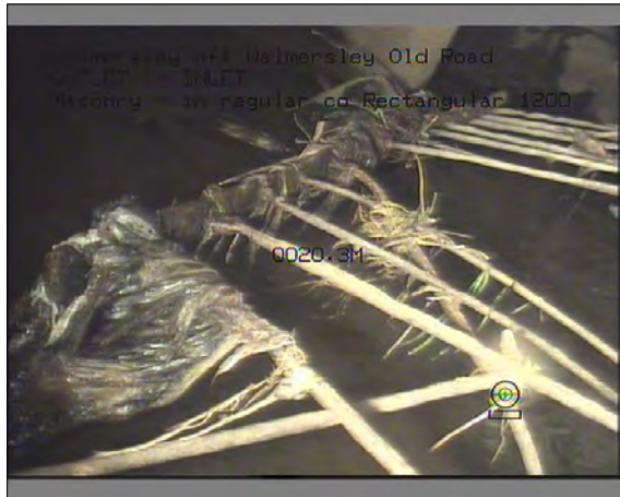
Photo: 017.JPG 20.3m, Settled deposits, other, 20% cross-sectional area loss
