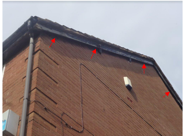
Fascia boards on most northern building. Significant gap between brick work and fascia board allowing access to internal cavity.
