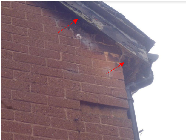
Northern elevation of most northern building. Obvious gaps between fascia board and brick work.
