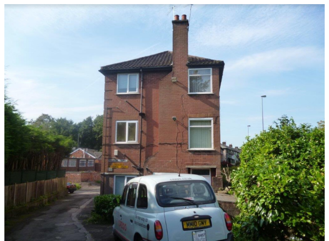
Southern elevation of the most southern building. Gaps between fascia board and brick work and also loose lead flashing around chimney breast.
