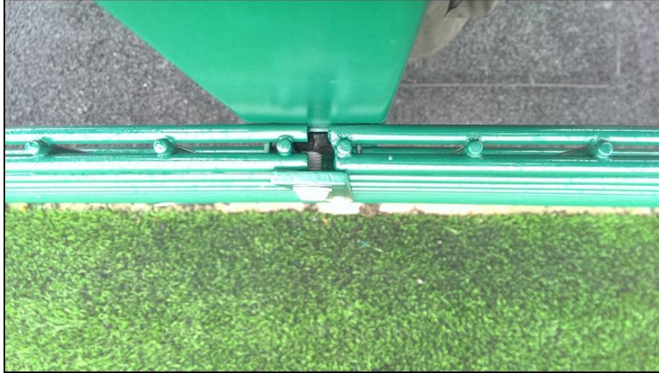
Figure 9: Image Showing Neoprene Isolators
