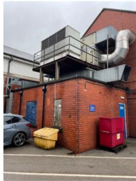
Poor quality building stock, ongoing maintenance drain, unsightly and defunct services
