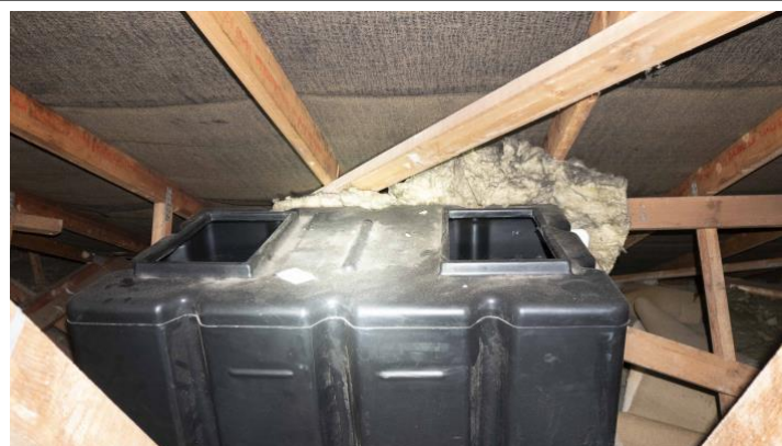
5. Cold water tank
