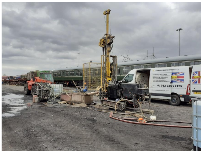
Borehole TDS 1A View south west
