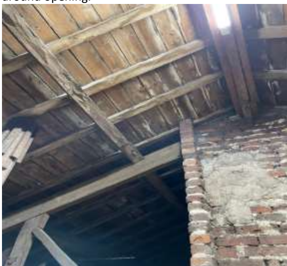
Evidence of water damage to timber boarding through water ingress and / or condensation.
