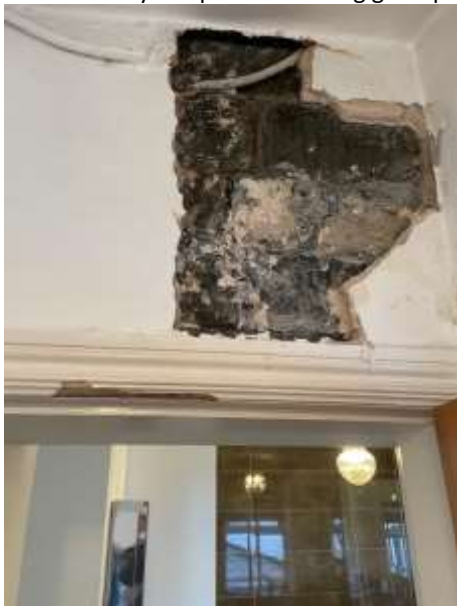
Evidence of water ingress from leaking roof above – with loose plaster removed to allow the masonry wall behind to dry. Water damage to timber architrave around opening.
