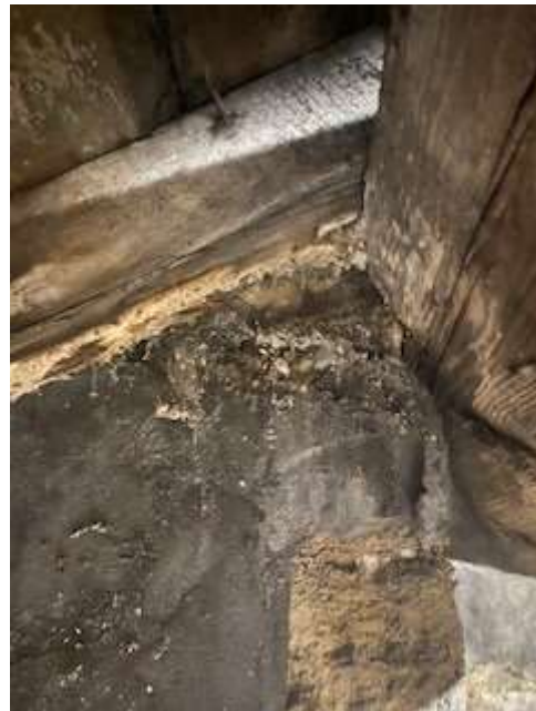
Evidence of some localised timber decay which requires further investigation and treatment by specialist timber treatment company.
