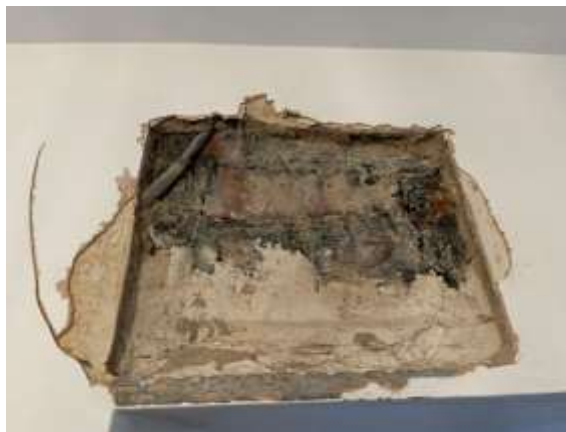
Evidence of water ingress from leaking roof above – with loose plaster removed to allow the masonry wall behind to dry out prior to making good plasterwork.
