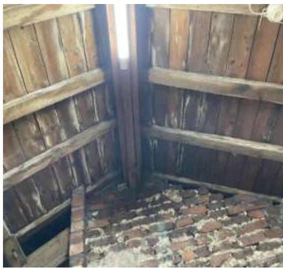
Evidence of water damage to timber boarding through water ingress and condensation forming on exposed galvanised clout nails.
