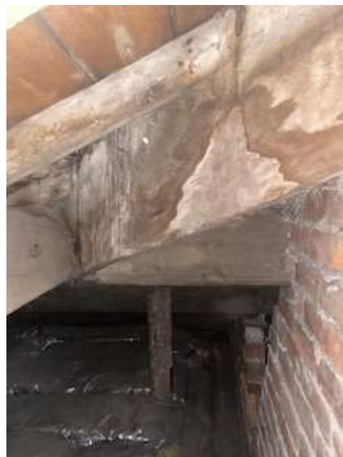
Evidence of water ingress onto timber purlins through roofing slates.
