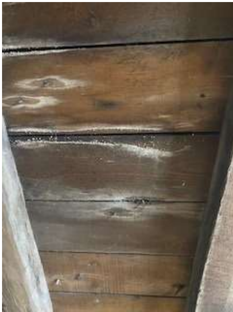
Evidence of water damage to timber boarding through water ingress and condensation forming on exposed galvanised clout nails.
