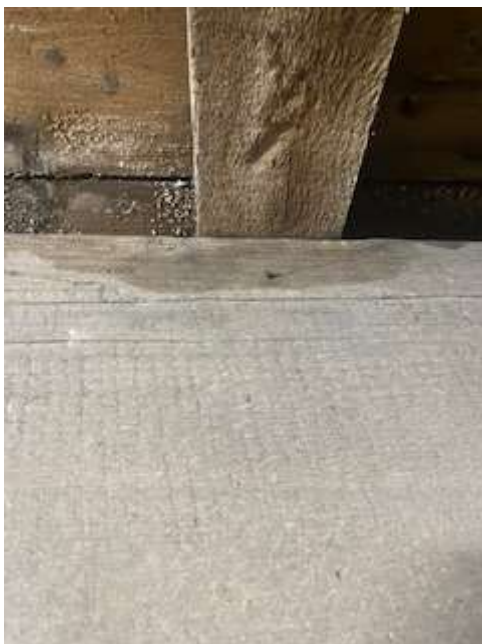
Evidence of localised mould growth following water ingress through roofing slates.
