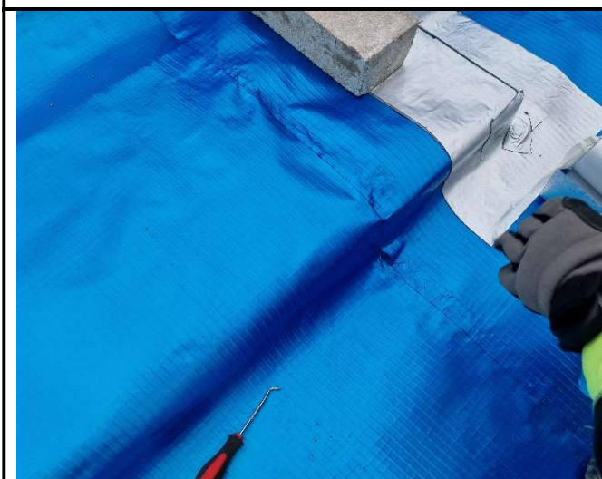
Figure 17 - Weak seam at interface VTcal to Horizontal
