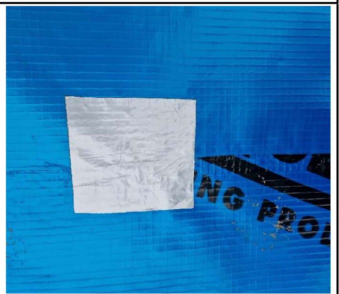
Figure 16 – Damage in Fig 15 patched with Visqueen Pro detail tape
