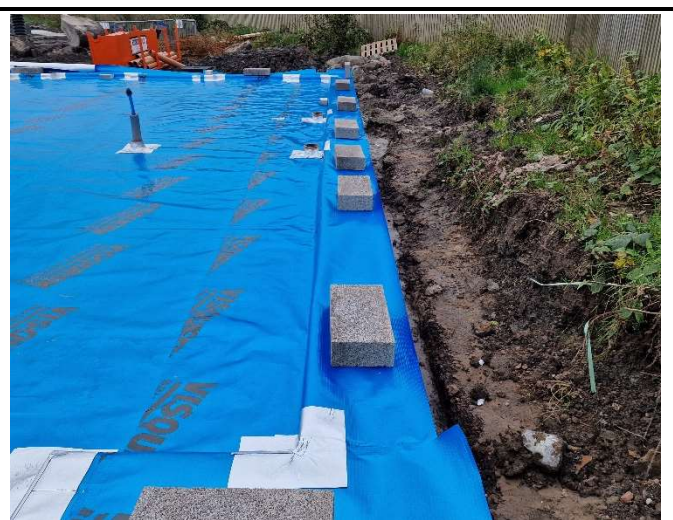
Figure 12 -- Cavities well covered
