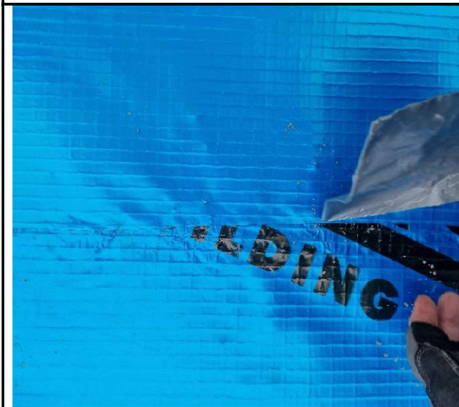
Figure 15 - Minor damage to membrane
