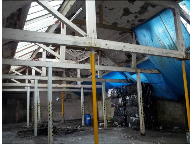
Plate 4. Interior of Building 1, looking south. Note debris from collapsed section of roof on floor.
