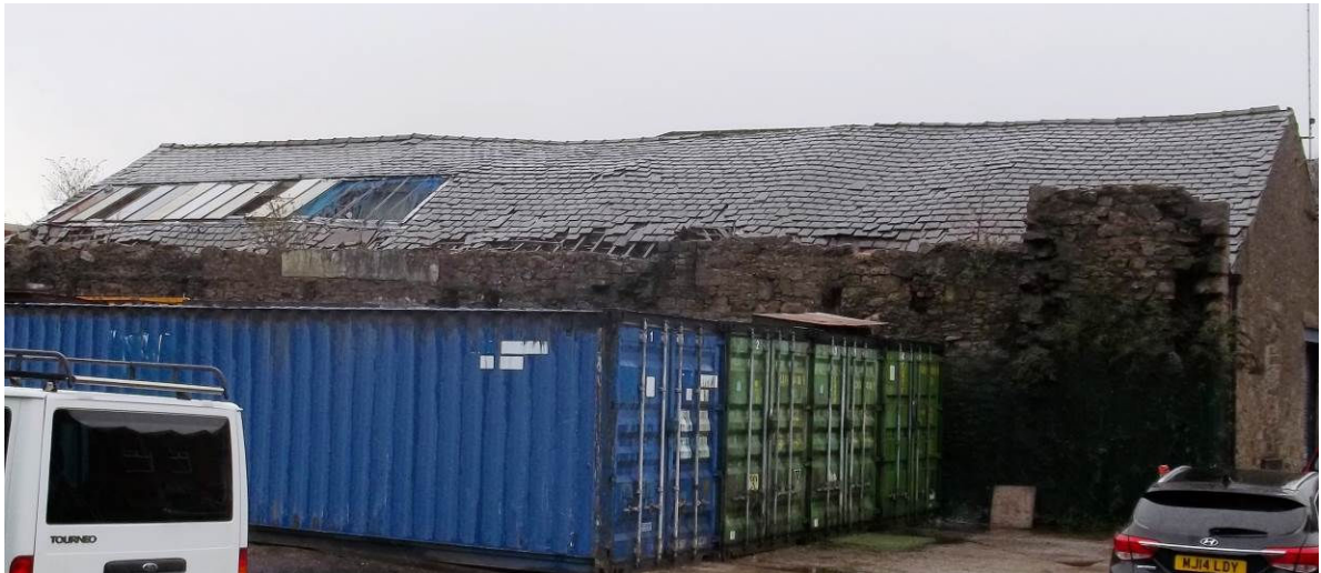
Plate 3. Eastern elevation of Building 1 showing uneven and missing slates.
