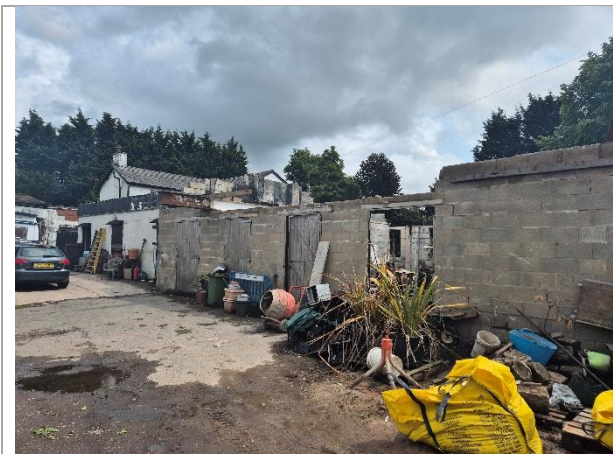
Photo 1: Hardstanding to the north of the burnt-out Workshop
