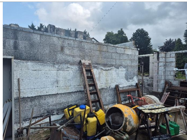
Photo 8: Concrete walls of the burnt-out Workshop
