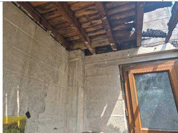
Photo 10: Concrete walls and section of former roof of the burnt-out Workshop
