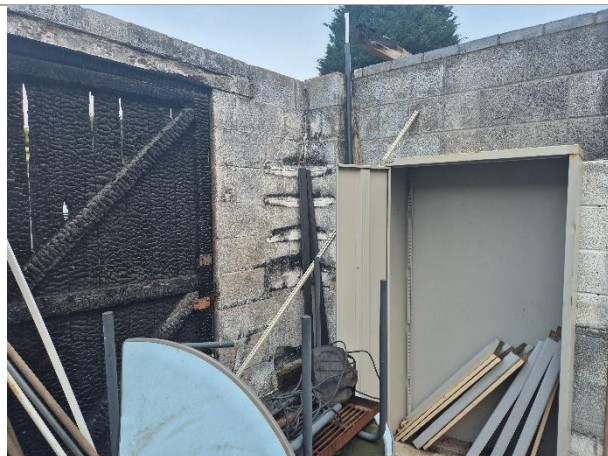
Photo 9: Concrete walls of the burnt-out Workshop
