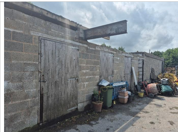
Photo 2: Northern elevation of the burnt-out Workshop
