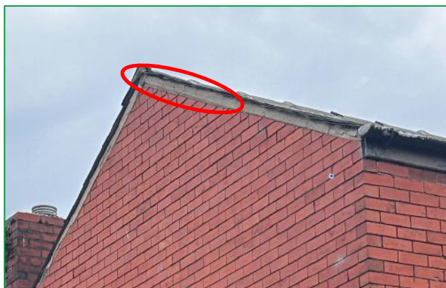
Showing crevices under slates on the northeast gable of Structure B
