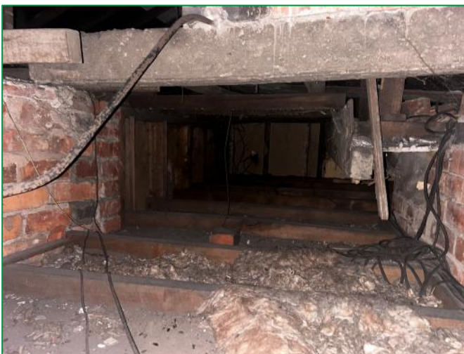
The loft void of Structure B – rat droppings are visible on the floor
