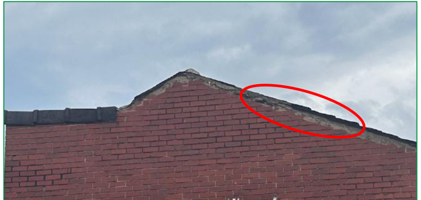
Showing crevices under slates on the northwest gable of Structure B
