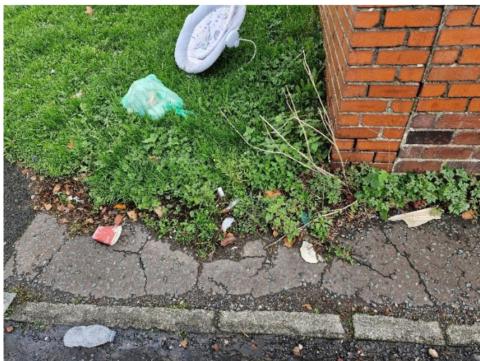
South east site boundary. Footway cracking, edgings required, kerbs misaligned/broken.
