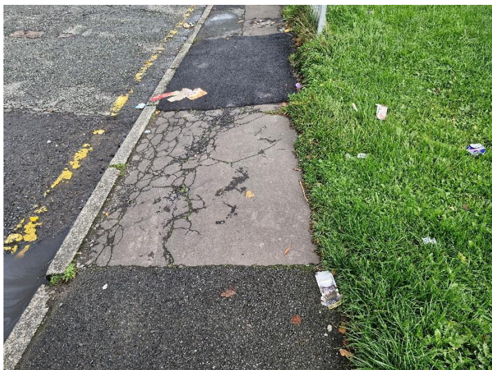
Footway on Chesham Rd showing relatively recent reinstatements and historical cracking.
