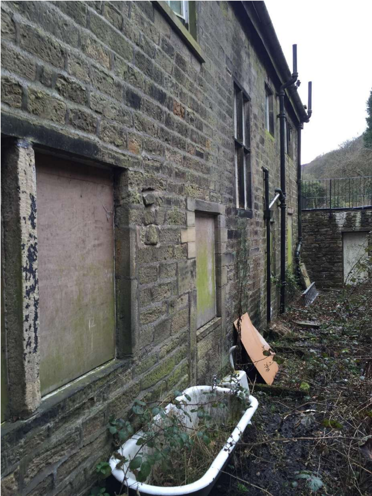
Figure 6. Rear elevation. Note alterations to original opening where stone has been built up to cill level but stone jambs and quoins remain.
