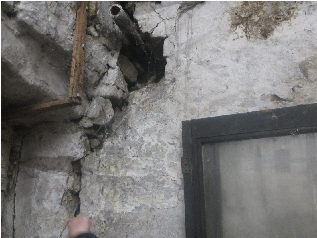
Photograph 22 – Large crack in the stonework identified during the internal inspection within Section A of Building 2.
