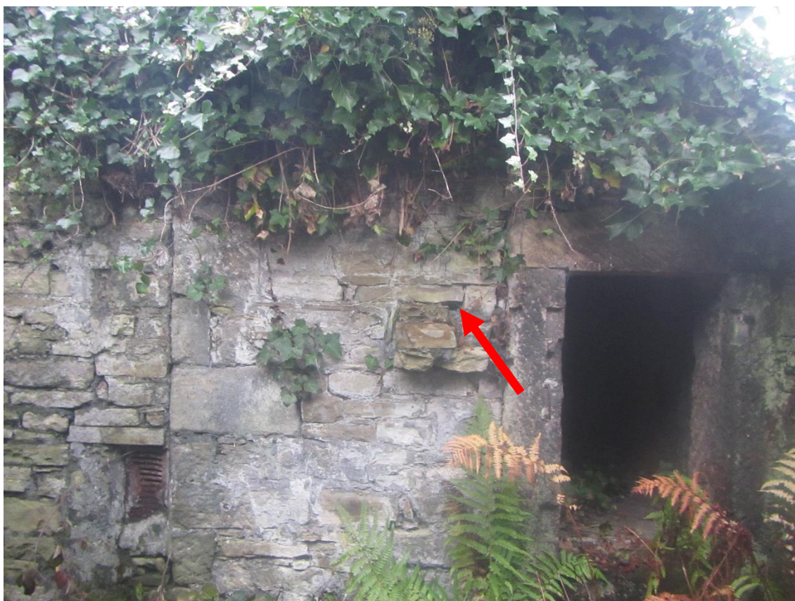
Photograph 3 – Southern aspect of Building 1, arrow pointing to gap in stonework.
