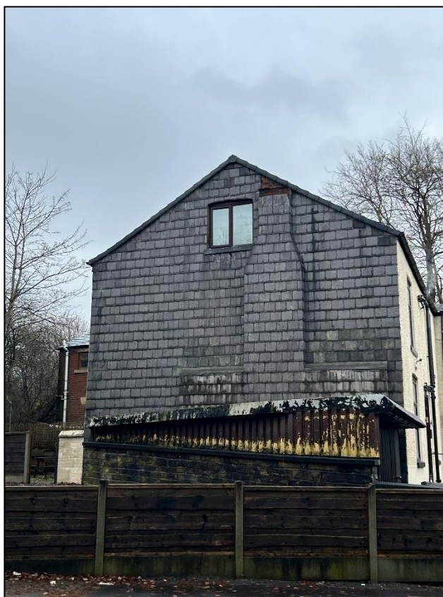
Plate 2 – The western aspect of the structure, note hanging slates
