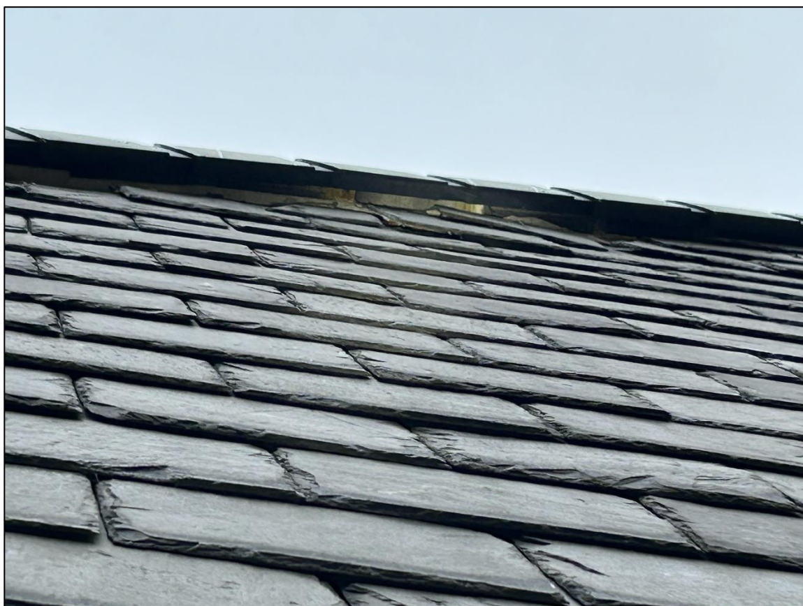
Plate 4 – Additional lifted hanging tile on western elevation
