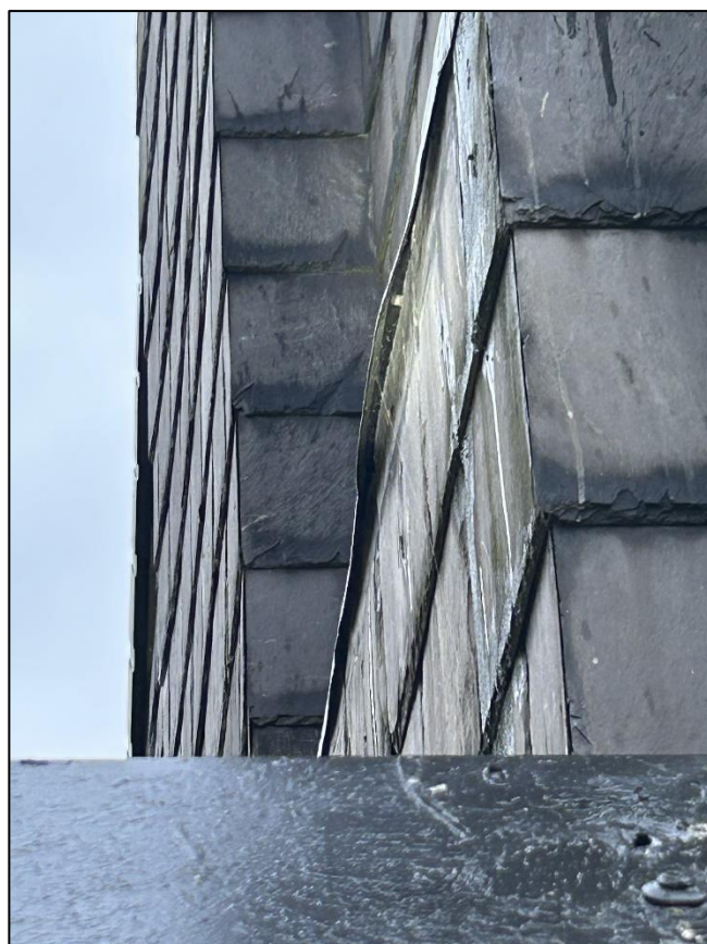
Plate 6 – Further area of lifted lead flashing on western elevation
