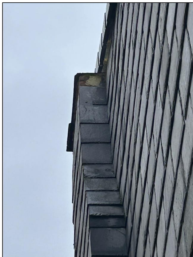
Plate 7 – Lifted and missing hanging slates on western elevation
