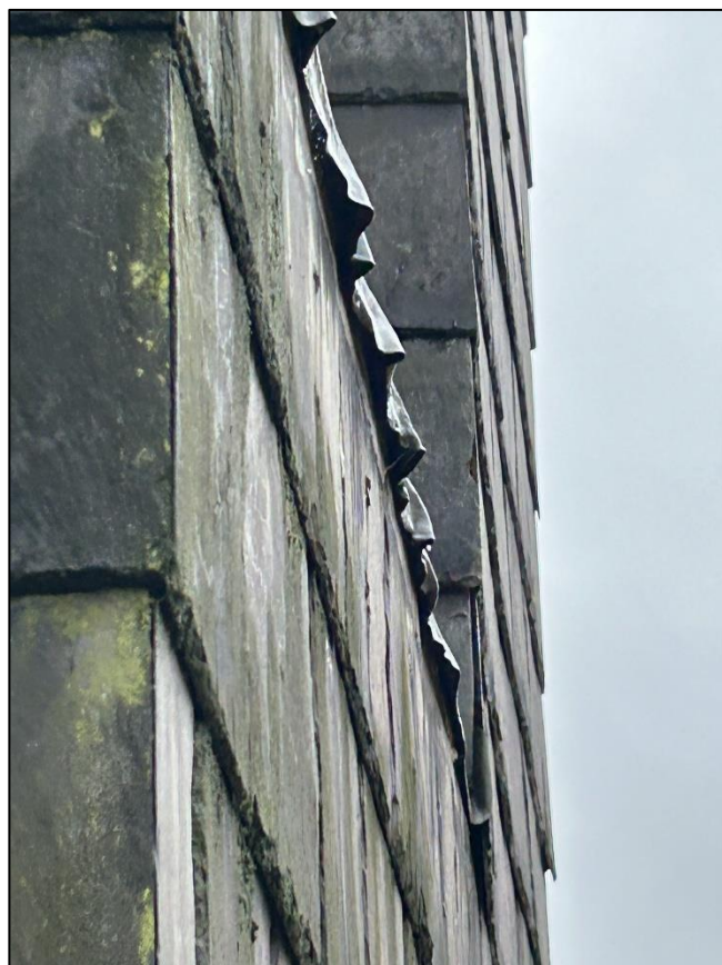
Plate 5 – Lifted lead flashing on western elevation
