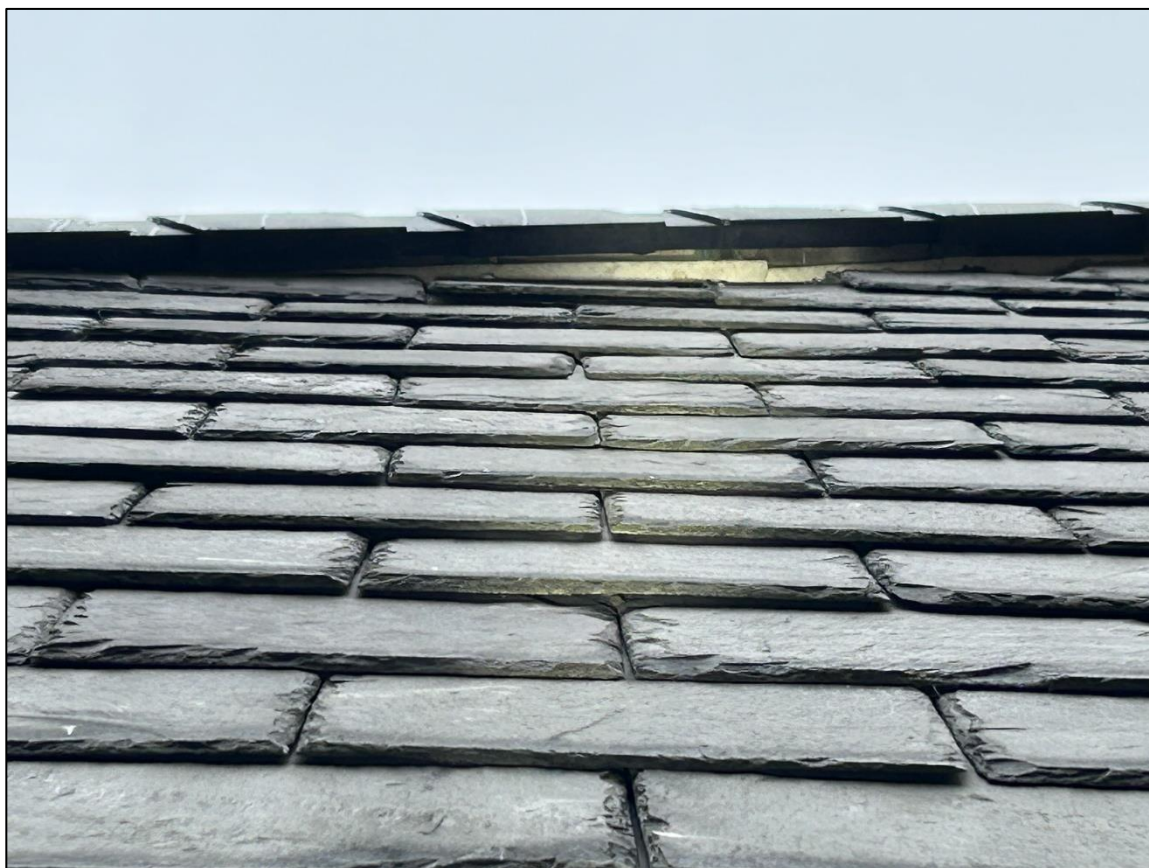
Plate 3 – Lifted hanging slate on western elevation and potential access into roof void at roof verge
